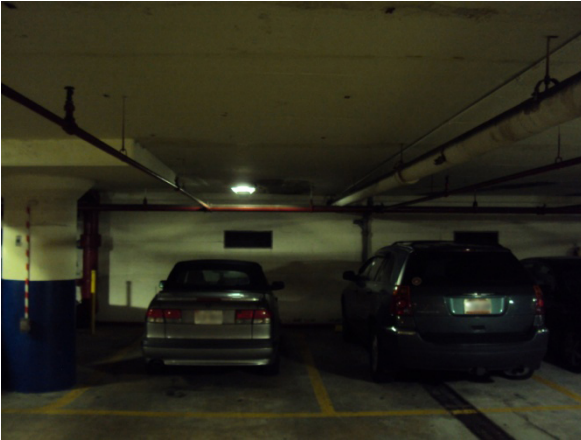
Figure 2.1. Occupied parking space with LED luminaire in low state (10% full power)
