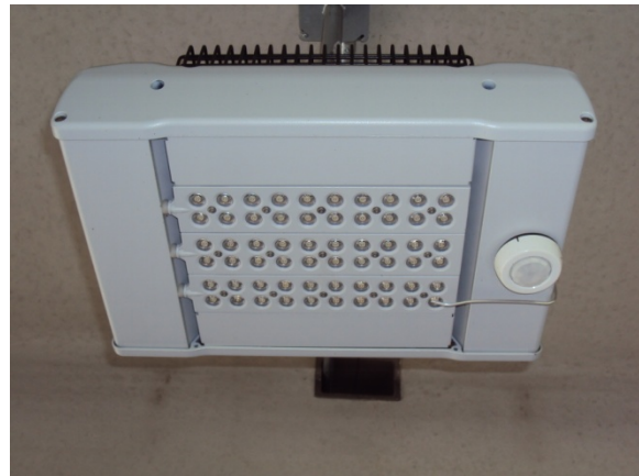
Figure 2.9. Close-up of LED luminaire and integral motion sensor (metering light pipe also shown)
