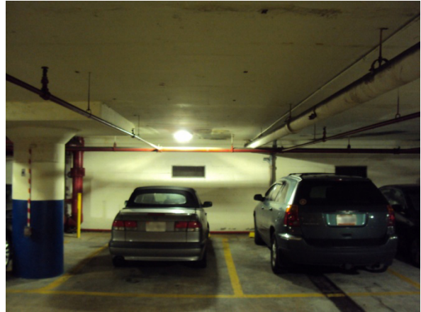
Figure 2.2. Occupied parking space with LED luminaire in high state (100% full power)
