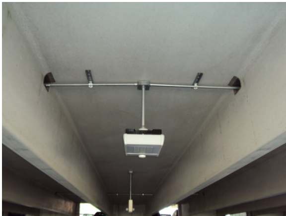
Figure 2.8. LED luminaire and pendant installation
