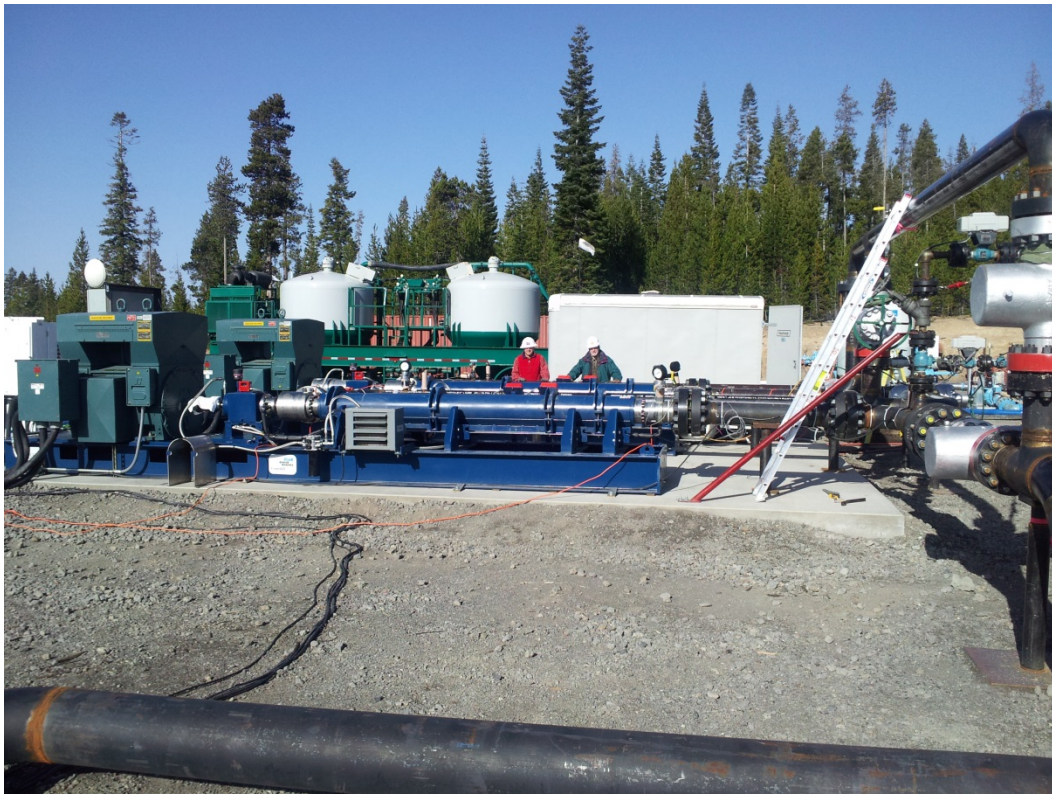
Figure 6.13. PNNL process trailer and mixing tank (top photo) used for tracer tests at Newberry Crater field site (bottom photo).
