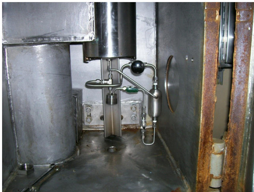
Figure 6. ANL's UV-visible spectroscopy equipment installed in-line with H Canyon sampler (hot sample aisle).
