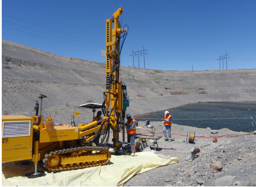
Figure 4. Photo of the direct push technology drill rig that was used during drilling and installation of the 100-C-7:1 temporary small-diameter well network
