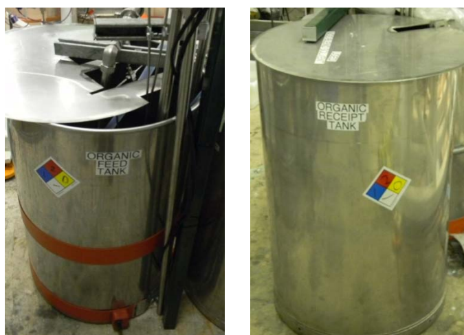
Figure 3-13. Side View of the Organic Feed (left) and Receipt (right) Tanks
