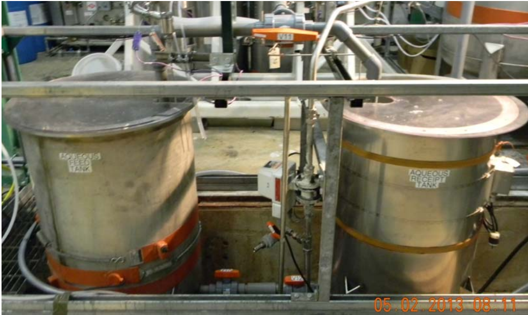
Figure 3-10. Side view of the Aqueous Feed (left) and Receipt (right) Tanks
