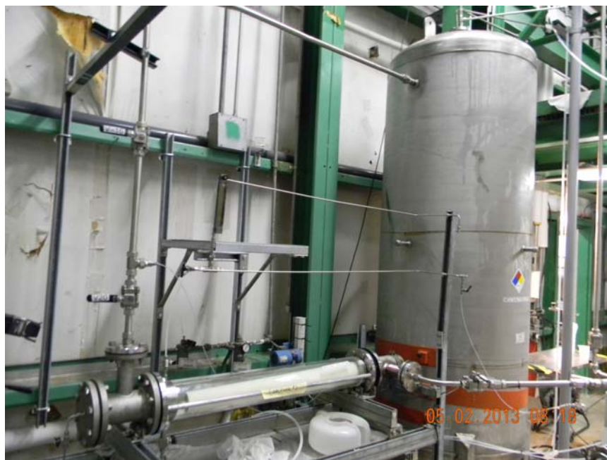
Figure 3-12. Coalescer, Lower Foreground, with 400-gallon Decanter in Rear
