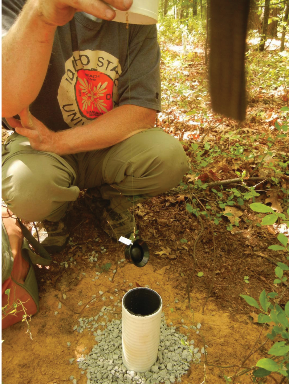
Figure 4. Installed measurement port with CR-39 detector being lowered into position.
