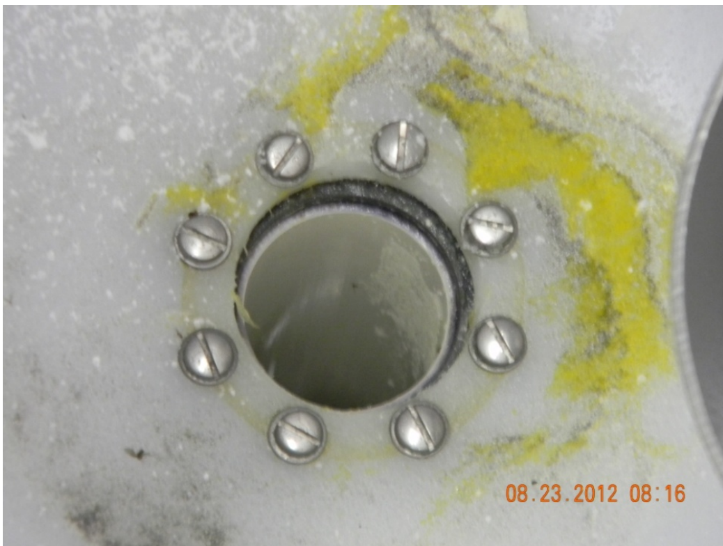
Figure 2-3. Close up of feed tank drain shown in the preceding figure.
