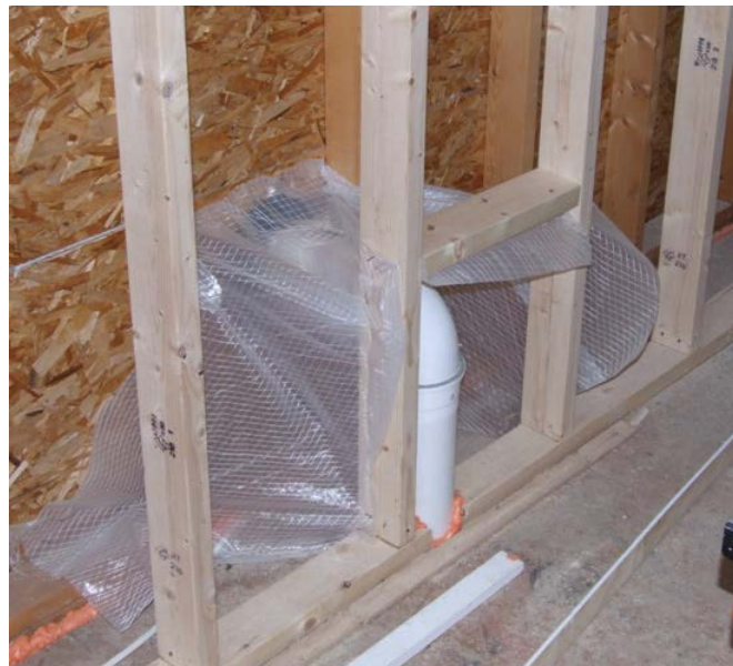
Figure 7. Insulation netting surrounding water heater combustion air and exhaust piping. These small areas were insulated separately to allow access if needed in the future.
