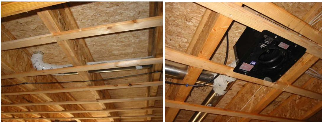
Figure 8. The exhaust fan and simple duct distribution system installed between the first and second floors.
