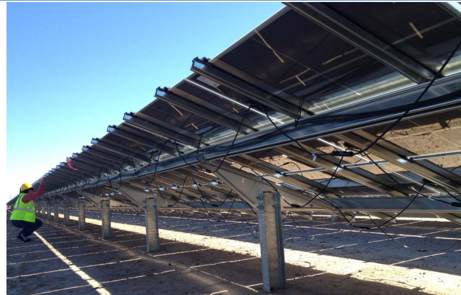
Field installation with poor (no) cable management
