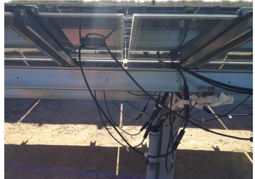
Detail of the cable routing. Photos courtesy of industrial partner.
