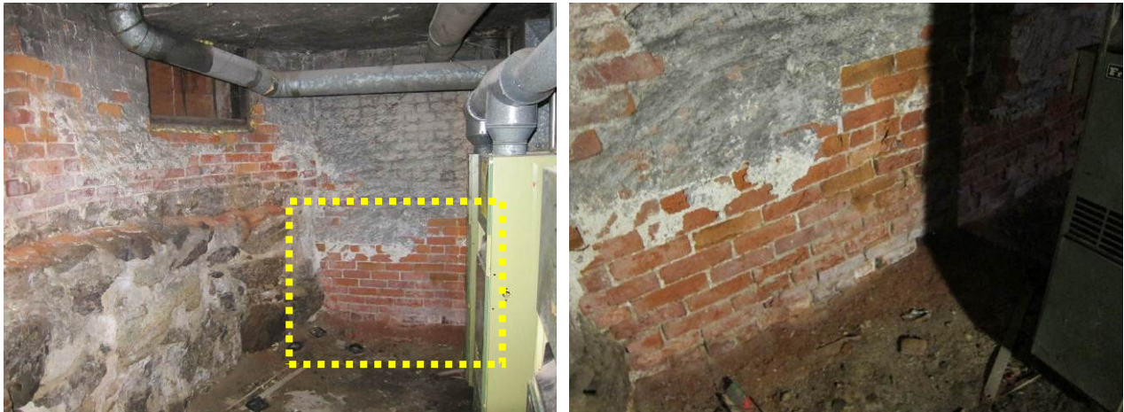
Figure 17. Capillary rise on south party wall (near furnaces). Left image shows front of building.
