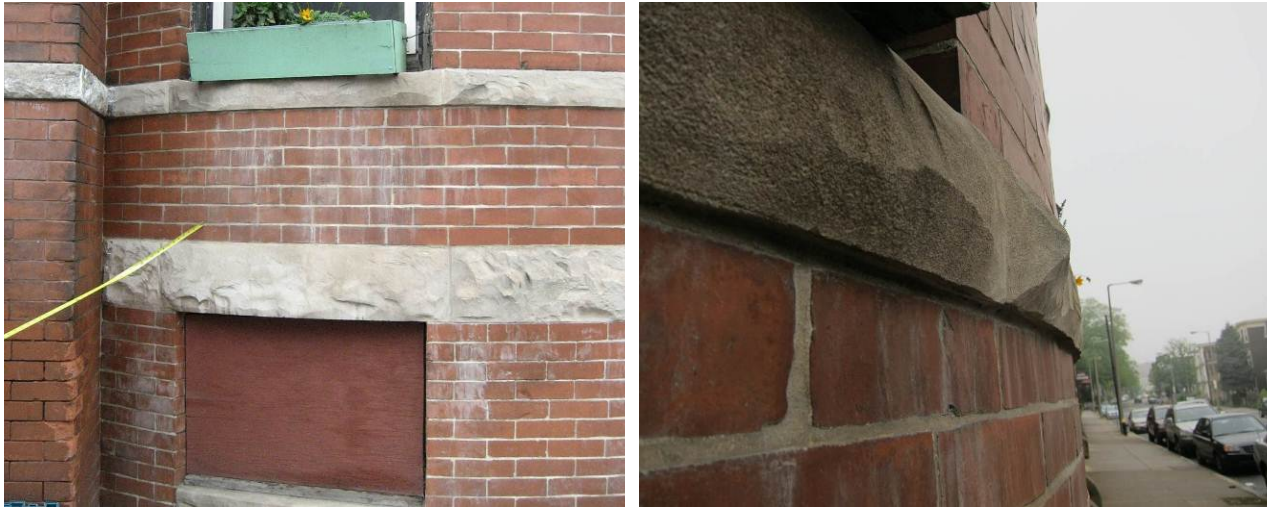
Figure 6. Efflorescence pattern under window sills (left); lack of drip edge at window sill band detail (right)
