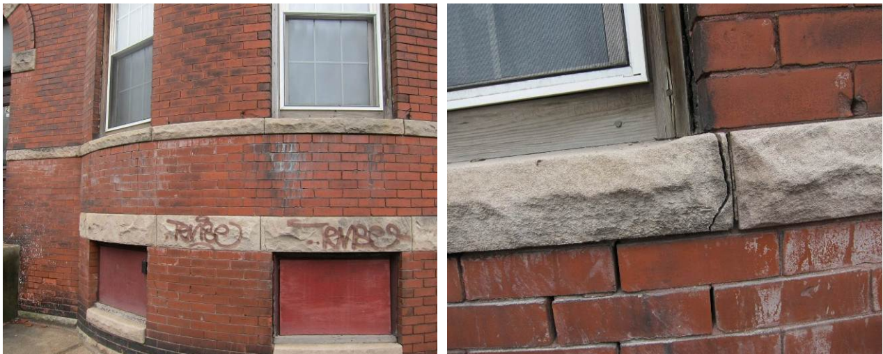
Figure 7. Adjacent building, showing severe mortar erosion under window sills
