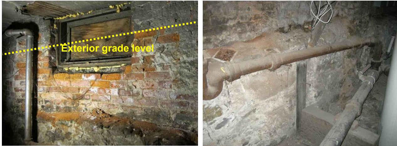
Figure 18. Severe subfluorescence at window at light well; stone shelf below grade
