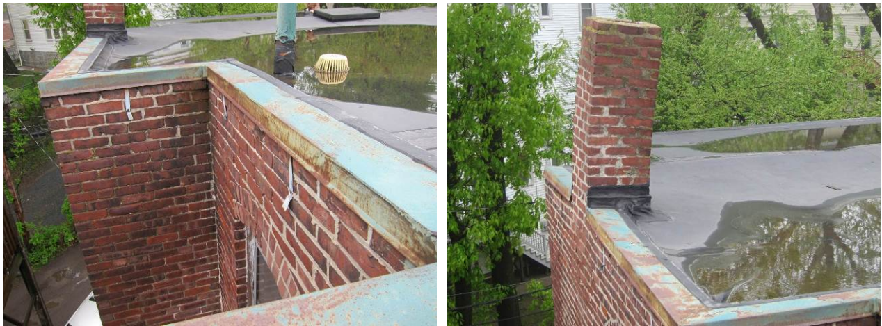
Figure 15. Brick condition at parapet near light well (left), and chimney condition (right)
