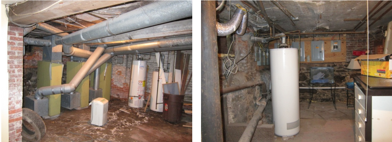
Figure 29. Gas furnaces (left) and DHW tanks (right)
