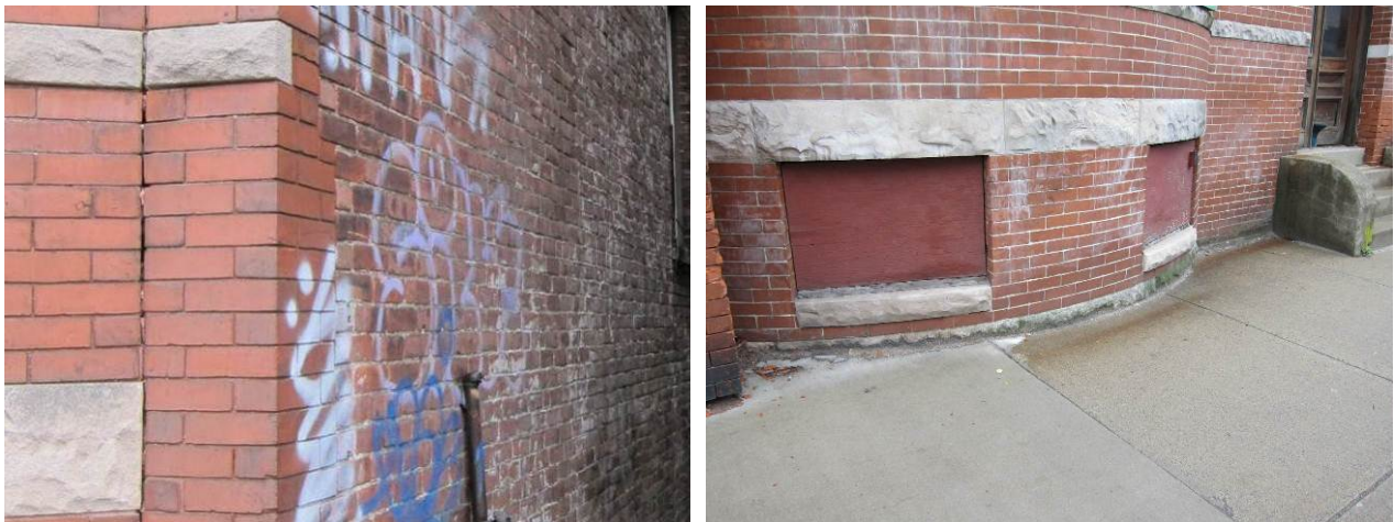
Figure 5. Front face brick/side brick transition (left) and brick termination at grade (right)
