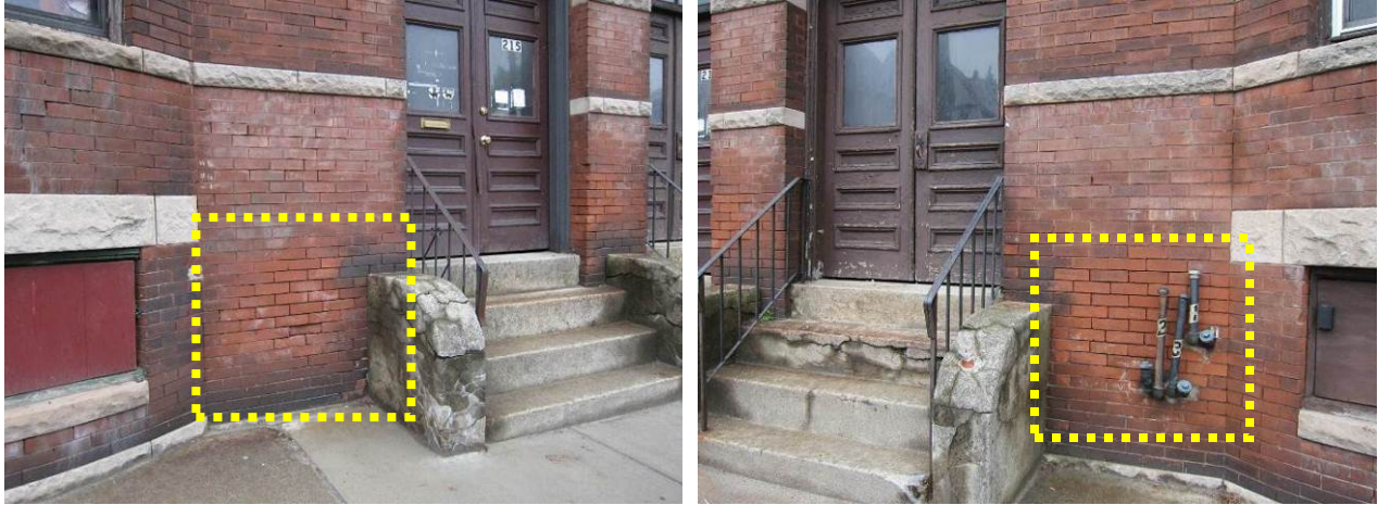
Figure 12. Freeze-thaw damage and mortar erosion next to front steps at two adjacent buildings
