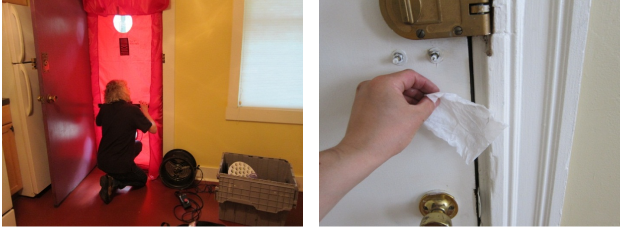
Figure 26. Airtightness testing; leakage at doors to hallway
