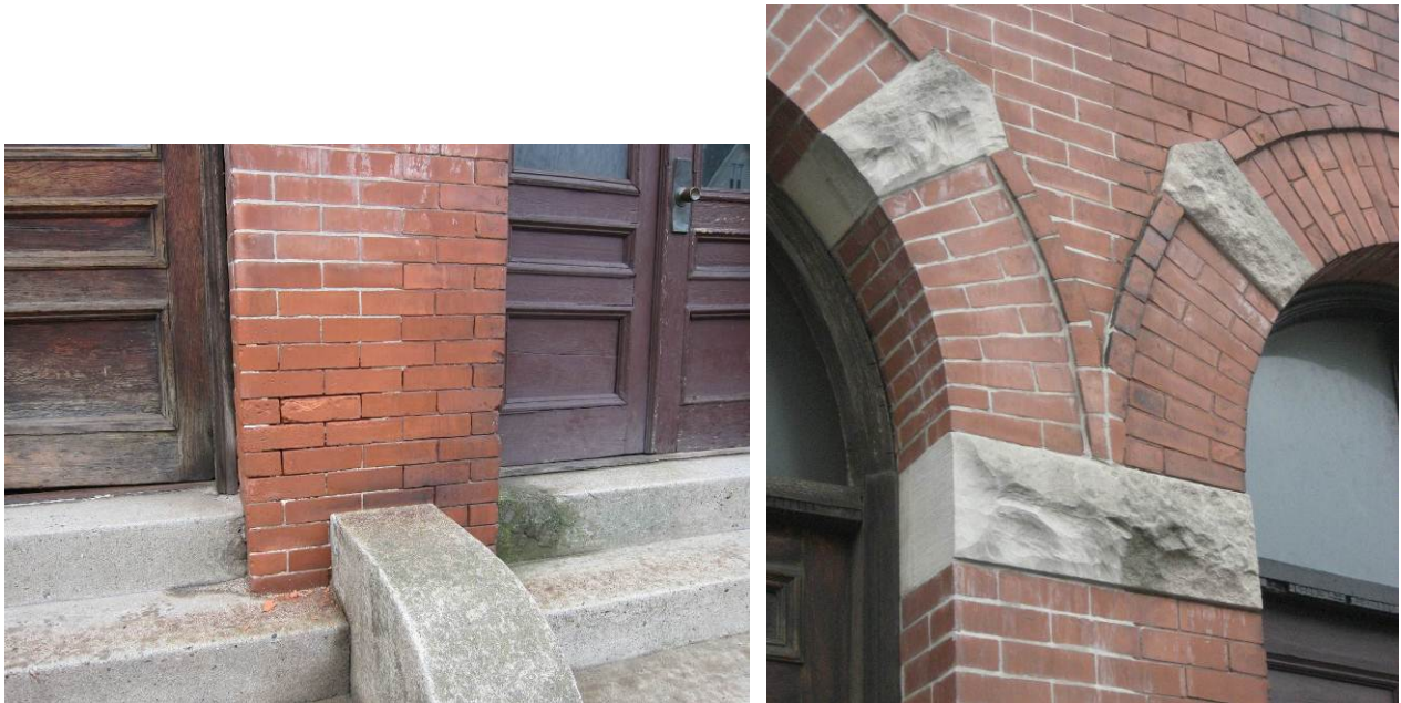
Figure 11. Freeze-thaw damage at front party wall (left) and doorway arch details above (right)
