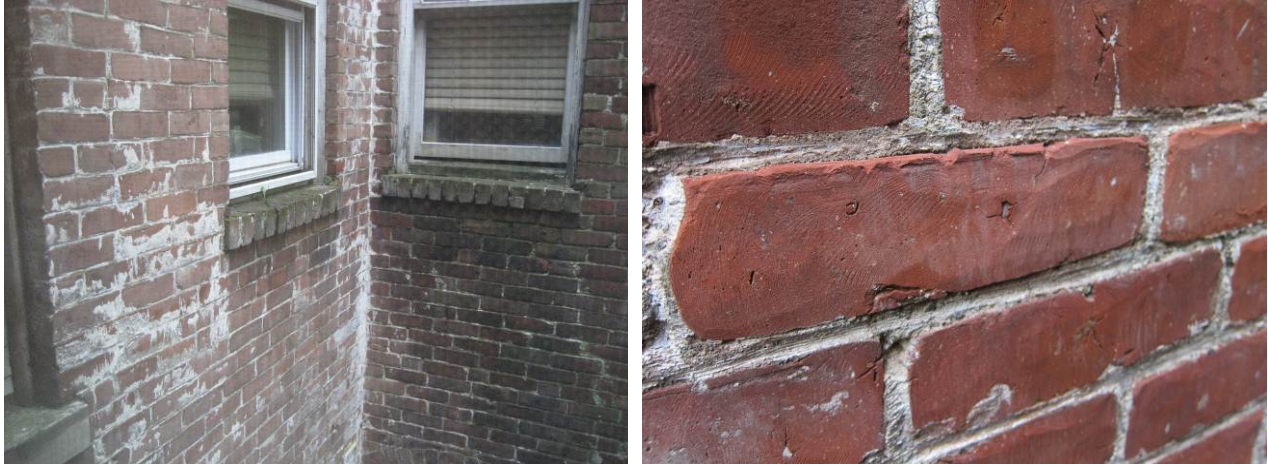
Figure 14. Residual paint at rear of building (left) and scarification of brick due to abrasive cleaning (right)
