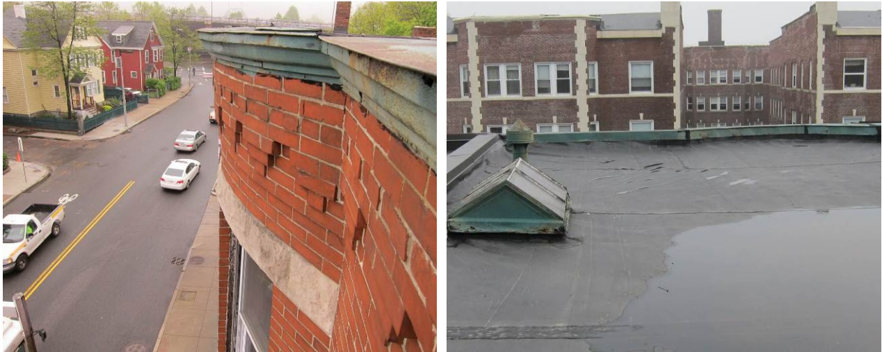
Figure 8. Front parapet brick condition (left) and interior side of parapet showing height (right)
