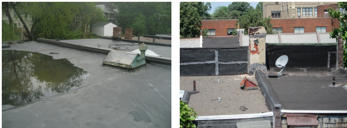
Figure 49. Capped party wall at J.P. Three-Family, and roof “wrap” over an exposed party wall
