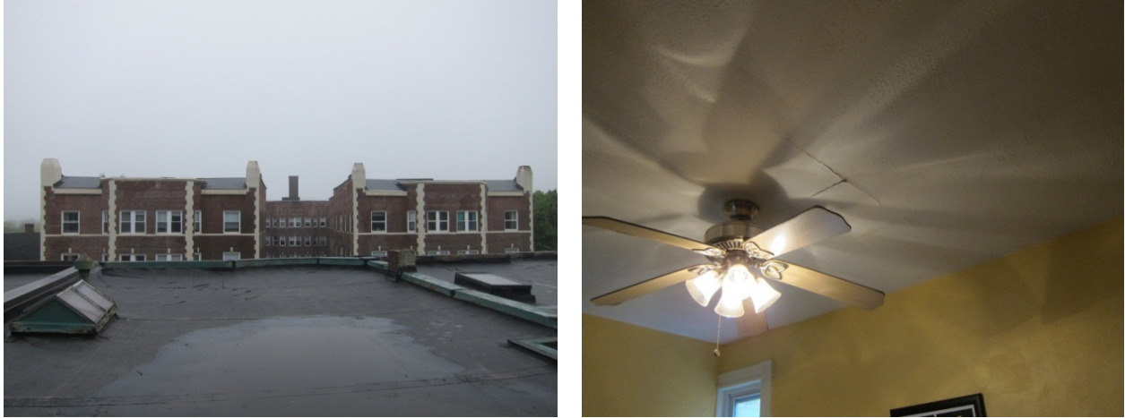
Figure 22. Rubber single-ply membrane roof and interior view of the third floor ceiling
