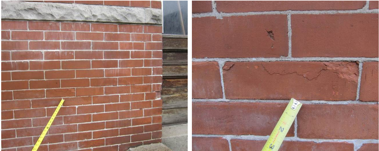
Figure 10. Minor freeze-thaw damage visible adjacent to front doorway
