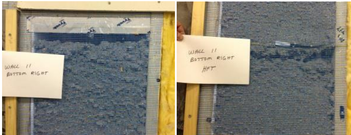
Figure 11. Gaps in wall cavities due to settling of cellulose, in the gypsum section of ‘Test wall 1’.
