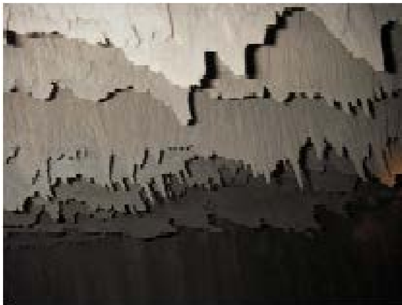
Fig. 6. Accumulation of low-melting temperature deposits on Schweinfurt low temperature screen tubes [12]
