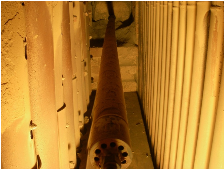
Fig. 45. Photo of the corrosion probe in the Gadsden power boiler just prior to its removal (photo courtesy of Billy Zemo, Southern Company).
