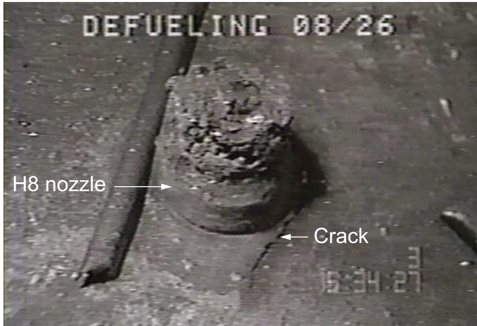
Figure 2-6. Video exams of the H8 instrumentation nozzle with crack on vessel.
