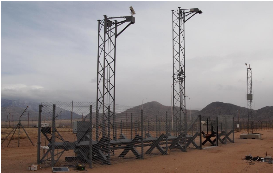
Figure 1: ReKon System Prototype Installation
