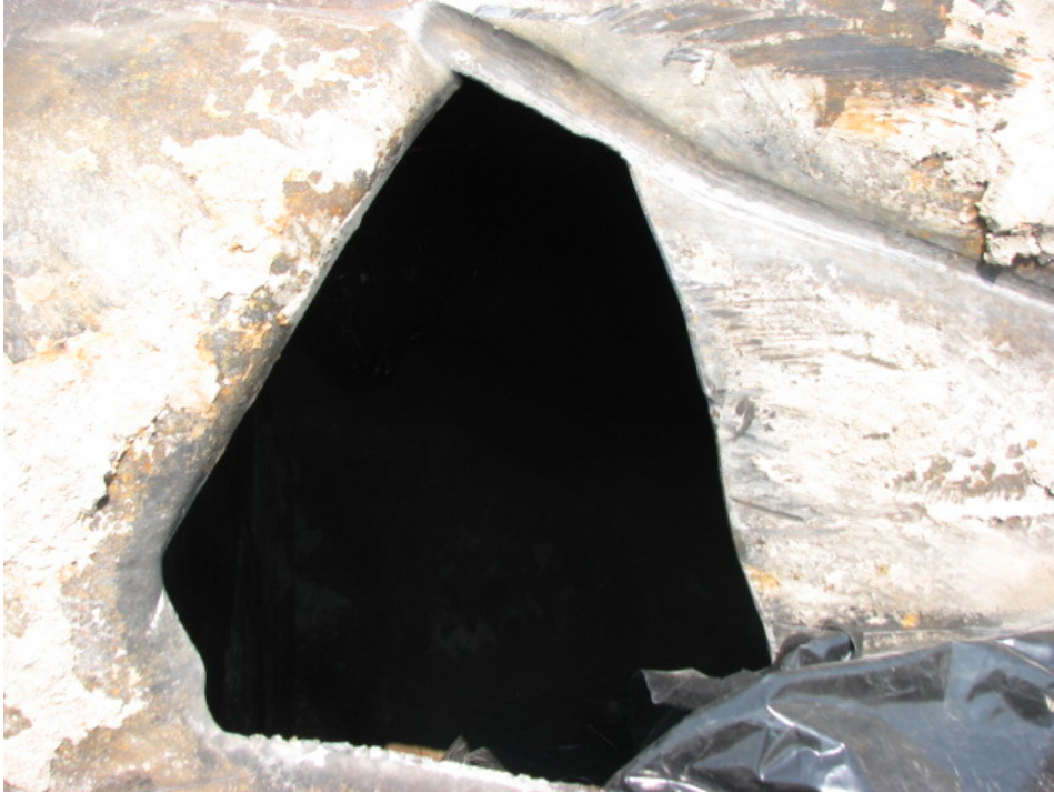
Figure 2 . Tank Rendered Unusable (holes punched in both sides)
