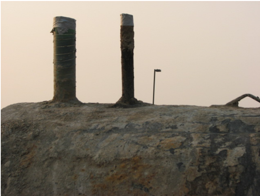
Figure 3. Tank Rendered Unusable (ports cut off)
