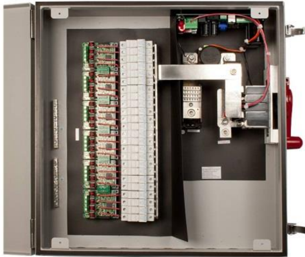
Figure 1: 24-String MidNite Solar combiner box with string level monitoring that was retrofitted to detect and mitigate series and parallel arc-faults.
