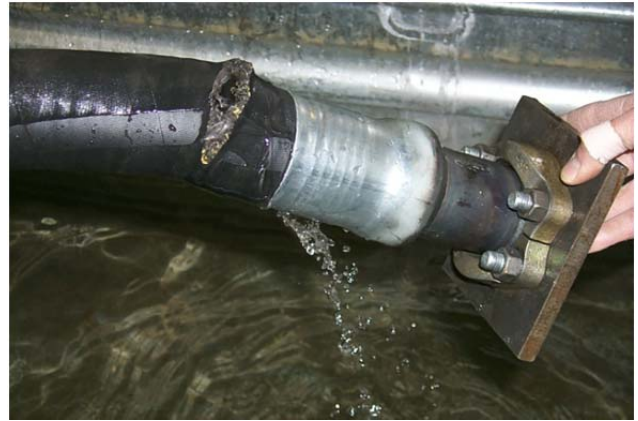
Typical hose failure near swaged end fitting
