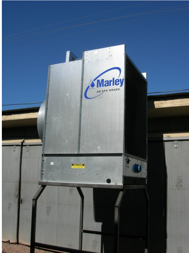
Figure 2-12. Evaporative Cooler. (The cooler has a name plate cooling capability of 220 kW.)
