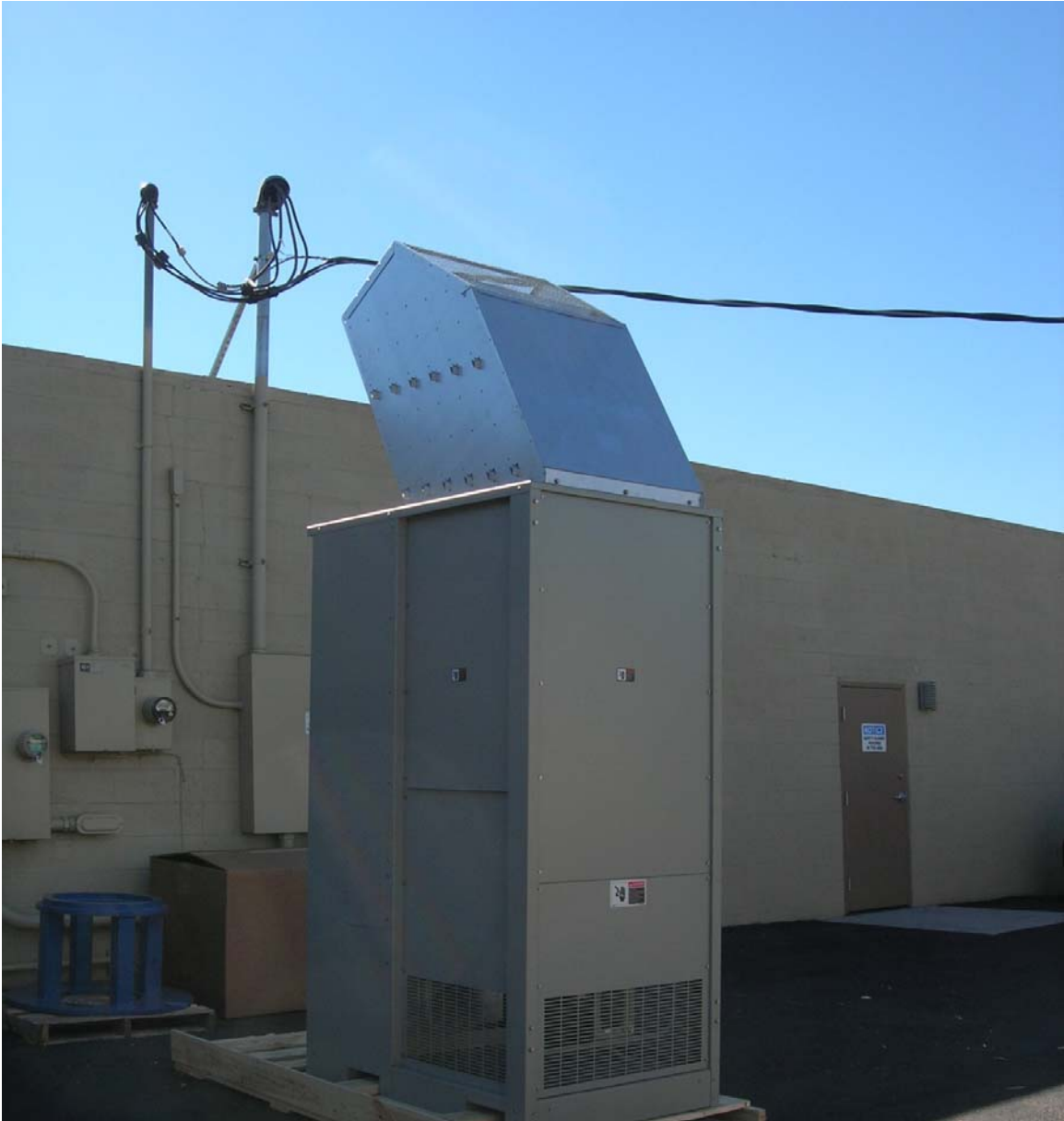
Figure 2-11. Avtron load banks.
