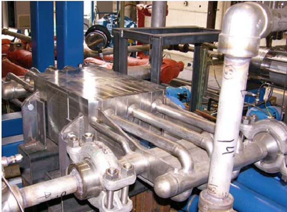
Figure 2-9. S-CO 2 LT PCHE recuperator.
