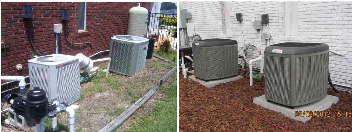
Figure 13. Heat pump compressors, pre- and post-retrofit
