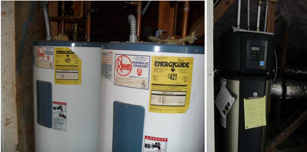
Figure 14. Electric resistance storage water heaters, pre-retrofit (left) and one of two electric HPWHs, post-retrofit (right)
