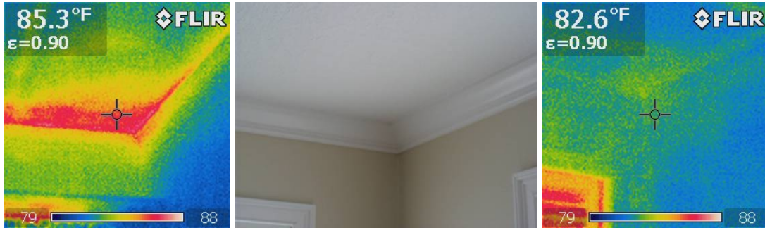
Figure 17. Wind washing of attic insulation at exterior wall corner in the master bedroom (left: pre-retrofit IR image, center: digital picture, right: post-retrofit IR image)
