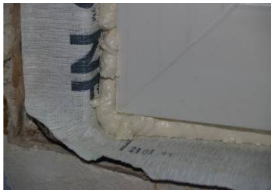
Figure 12. Foam sealant at window unit interior [Image courtesy of BARA]
