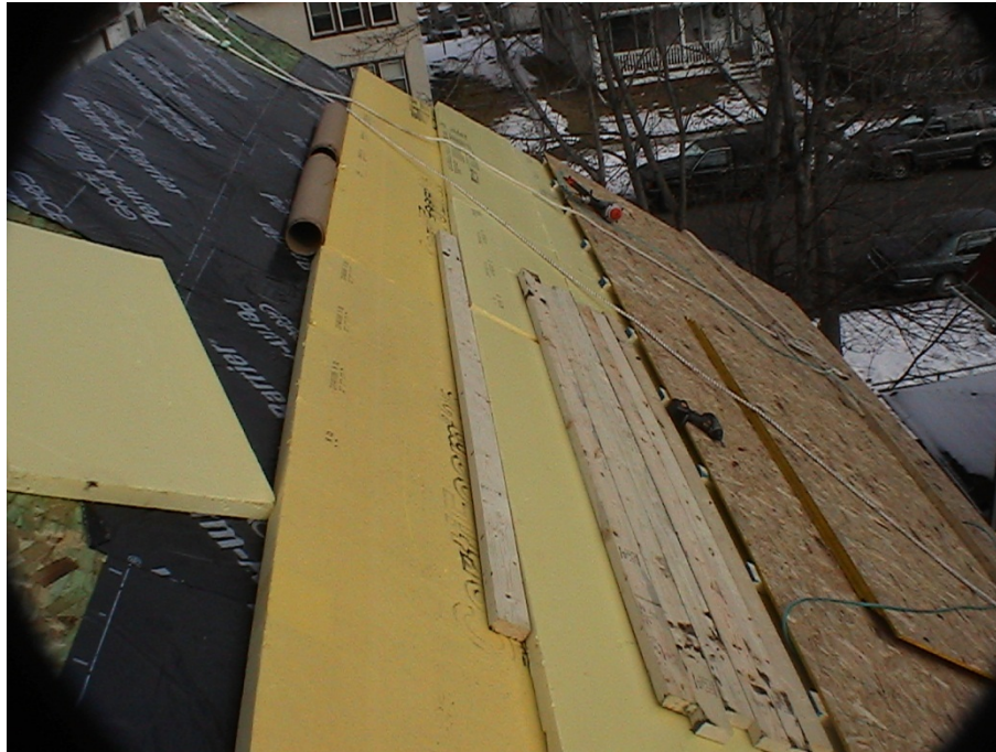
Figure 4. Details of ETMMS exterior overcoat retrofit on 1½-story home (Courtesy of Cocoon)
