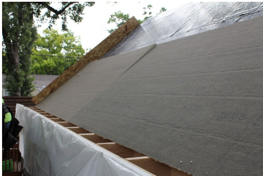
Figure 25. Transition where new insulation meets eave wall and new soffit (Courtesy of Cocoon)
