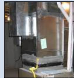
Figure 5. Sheet metal supply plenum
