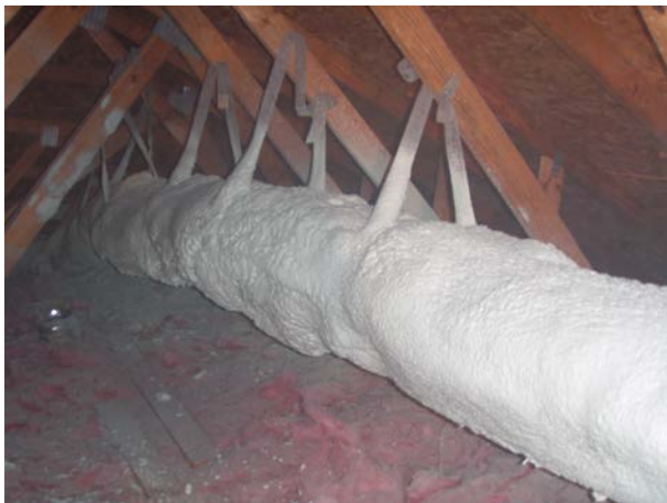
Figure 6. Encapsulated duct in attic
