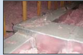
Figure 4. Fiberglass duct board ducts in an attic
