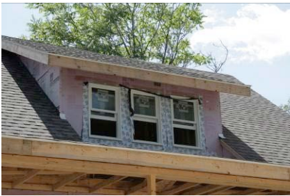
Windows above front porch requiring remediation
