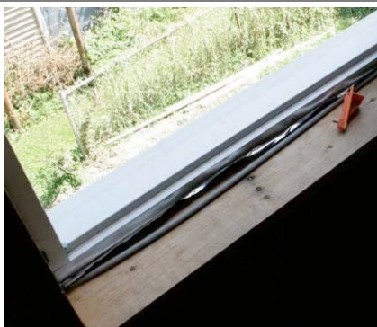
2011-08-28 – Backer rod back-dam failing to adhere to the flashing tape
