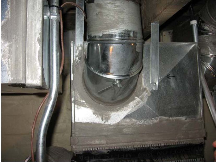
Figure 14. Typical ductwork sealing at takeoff from trunk; elbow to the site is sealed
