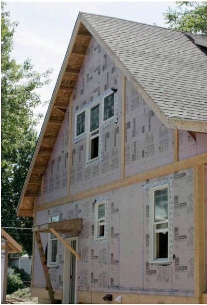
Areas where flashings below the windows need to be removed
