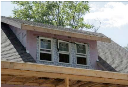
Windows above front porch requiring remediation
