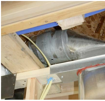
Venting hole requiring foil tape repair
