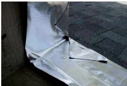
2011-08-28 – Gap in corner flashing
