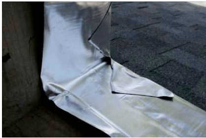
2011-08-28 – Gap in corner flashing
