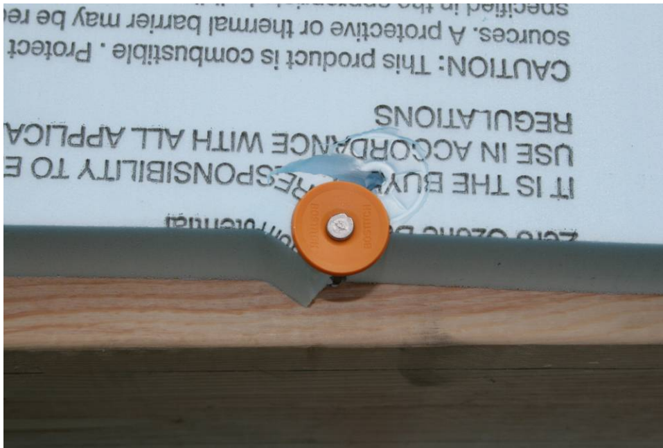
Figure 23. Nail pulling through XPS
