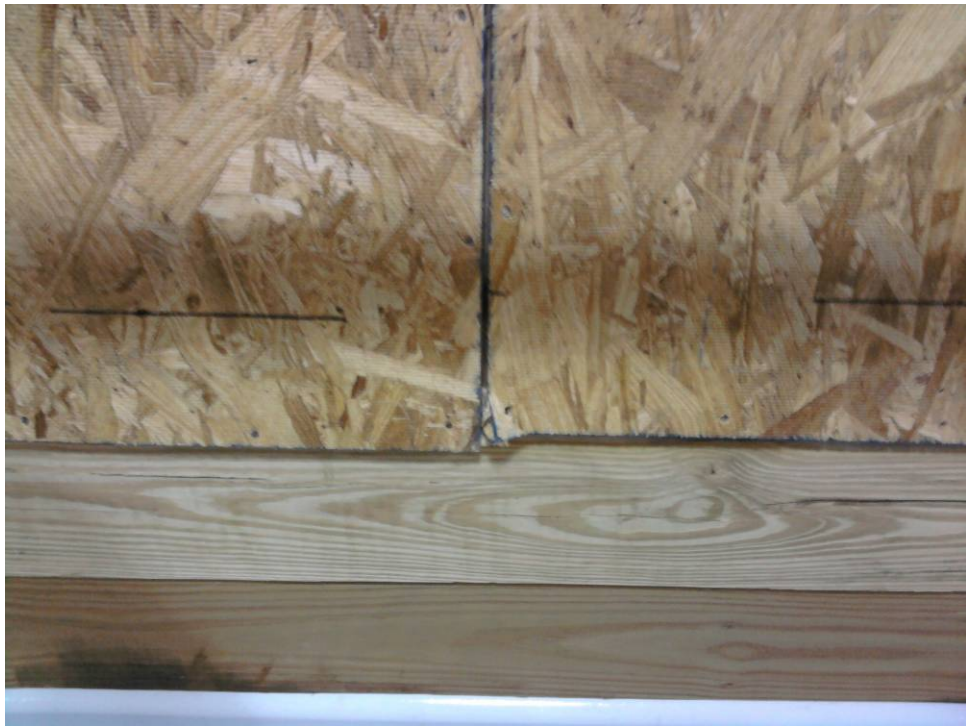
Figure 19. OSB failure at fastener
