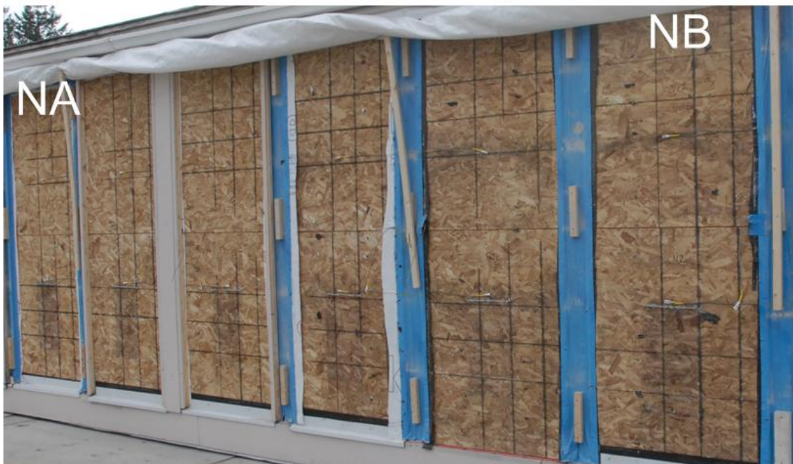
Figure 47. Exterior OSB sheathing on the north orientation immediately following deconstruction (photo taken from the opposite direction of Figure 46)
