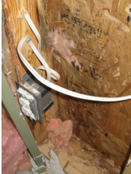
Figure 39. Example of air leakage condensation durability issues
