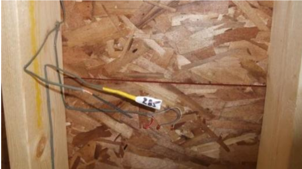
Figure 29. RH and temperature sensor installed in a stud bay (with MC pins installed below)
