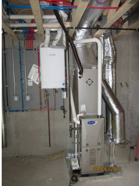
Figure 12. Air handler in basement
