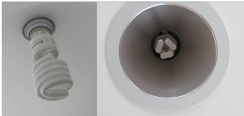
Figure 10. CFL and pin-based lighting installed
