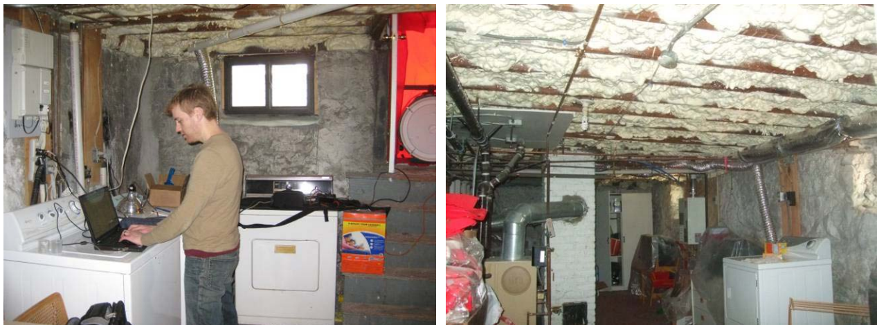
Figure 3. Arlington, MA, duplex basement ceiling spray foam, and nullled air leakage testing
