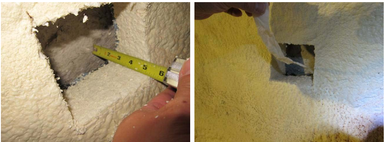
Figure 53. Air gap behind membrane; demonstration of airflow behind foam, Westford Barn/House
