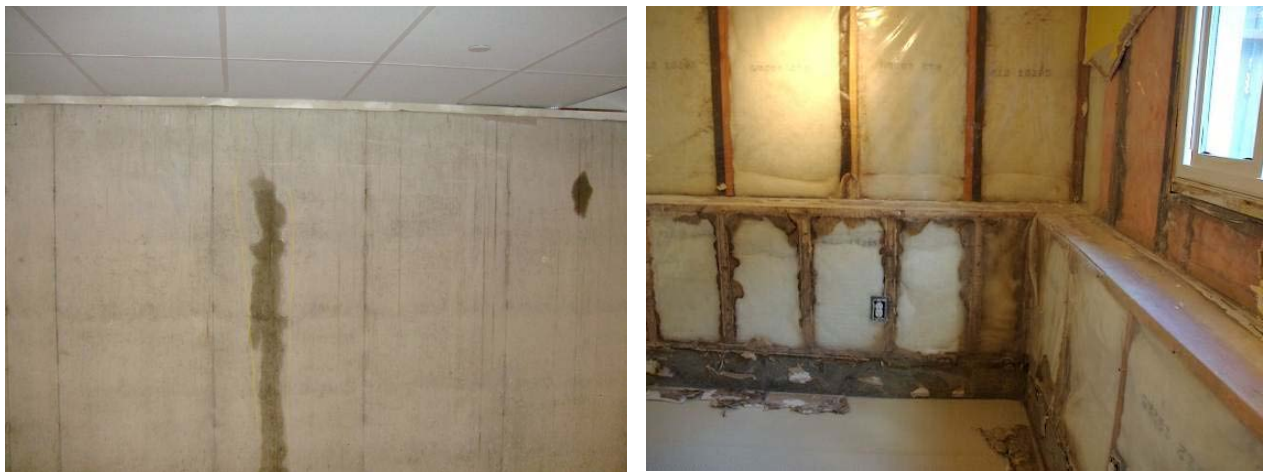
Figure 1. Active seepage through cast concrete (L); water damage concealed behind finishes (R)
