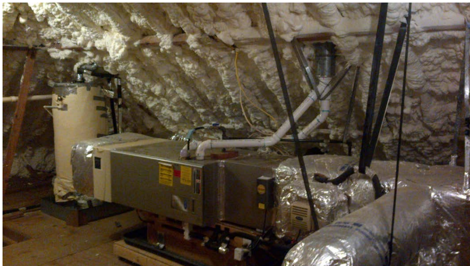
Figure 1. Non-vented attic houses equipment and ducting
