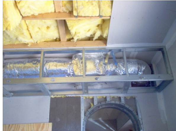
Figure 2. Duct chases in conditioned space
