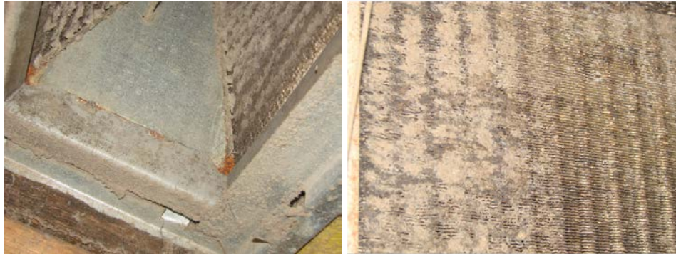
Figure 19. Looking up at pre-retrofit clogged, dirty cooling coils in the AHU (left); corroded and clogged cooling coil (right)
