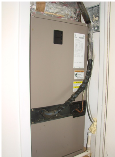
Figure 31. Crowded AHU closet with little room to access and seal duct connections to cabinet
