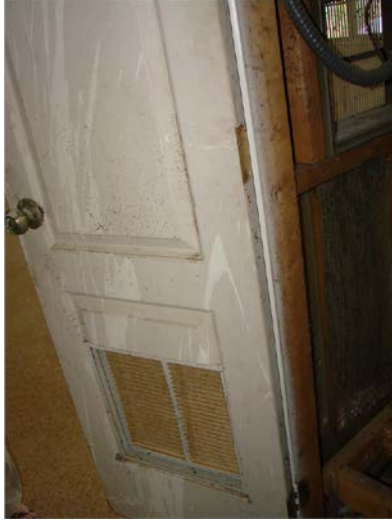
Figure 26. Interior closets that served as return plenums had louvered doors or door-mounted return grilles.
