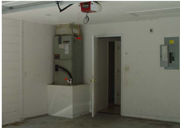
Figure 27. Upflow AHUs on framed platforms in garage with a wall-mounted filter-back grille were ducted directly into the platform cavity.
