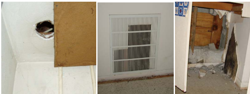
Figure 16. Pre-retrofit drywall penetrations: The ceiling fixture was removed, but penetration to the attic was unsealed (left); plumbing access in the wall covered with a return grille rather than a solid cover or patch (center); large opening beneath the bathroom vanity where block and drywall were removed as part of an incomplete renovation (right).
