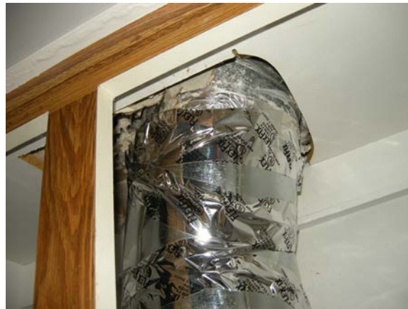
Figure 18. Post-retrofit: Unsealed range hood penetration through top of cabinet into the attic
