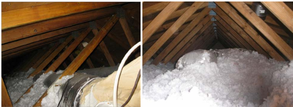
Figure 14. Post-retrofit ducts buried by blown-in fiberglass
