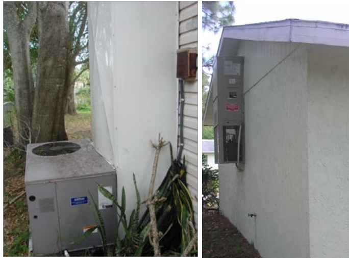
Figure 29. Exterior package units with return air path through a wall-mounted filter-back grille. Ground mounted unit with metal shroud housing main return and supply ducts (left) and wall-hung unit with attic-mounted ducts (right).
