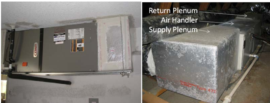
Figure 28. Horizontal flow AHUs mounted at ceiling of garage (left) and in the attic (right)
