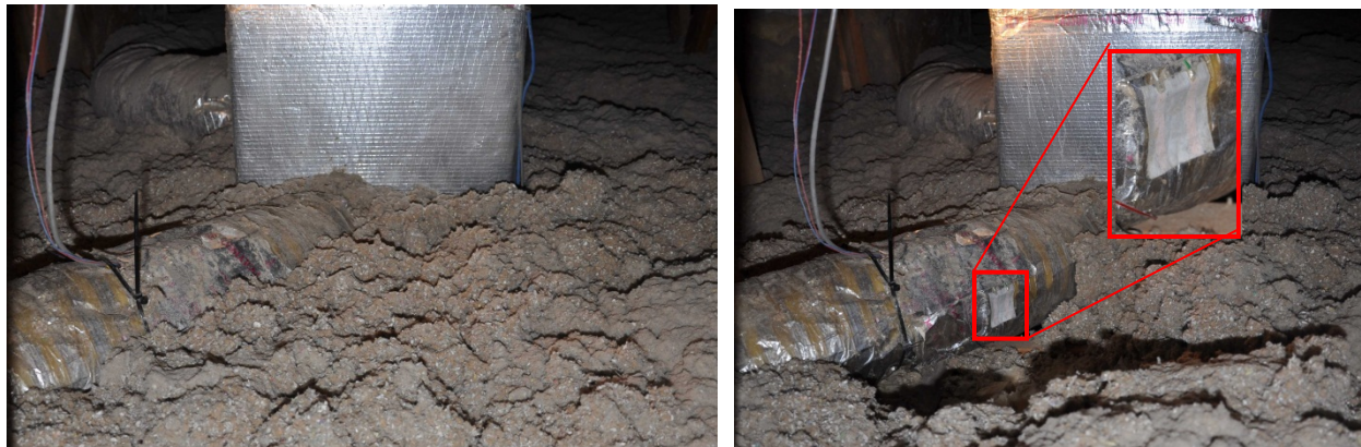
Figure 2. Photos of buried duct (left) and exposed moisture sensing strip (highlighted, right)
