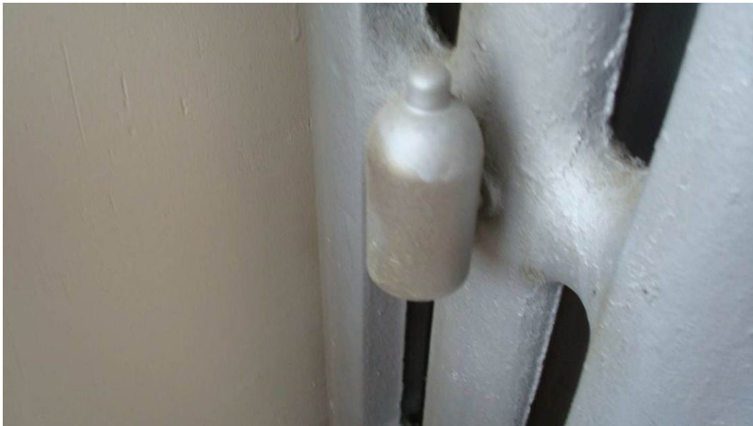
Figure 12. Painting over radiator vents is a common oversight that can have a serious effect on the heating in an apartment. Blocked radiator vents must be cleaned or replaced.
