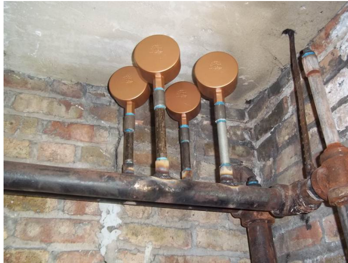
Figure 5. Main line air vents installed on a steam line.
