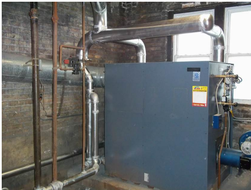
Figure 2. A cast-iron sectional steam boiler in good working condition in a building that could benefit from balancing
