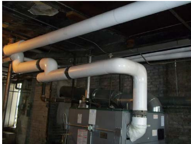
Figure 8. Insulated heating pipes (used with permission from CNT Energy 2011)
