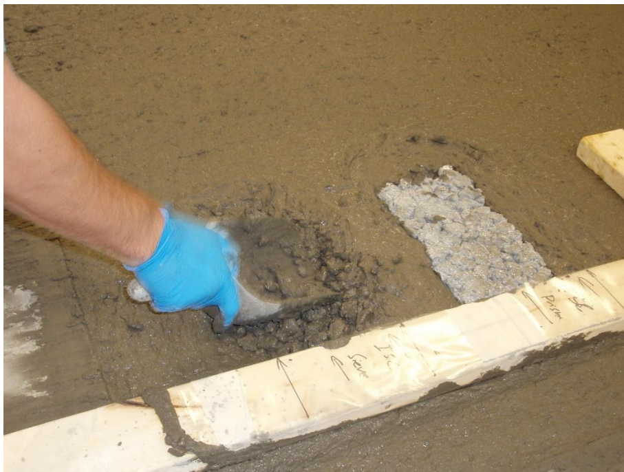
Fig. 15. Installing wet-sieved concrete into the surface to more realistically simulate poor consolidation.
