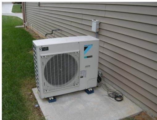
Fig. 3. The Daikin inverter compressor at CC3.
