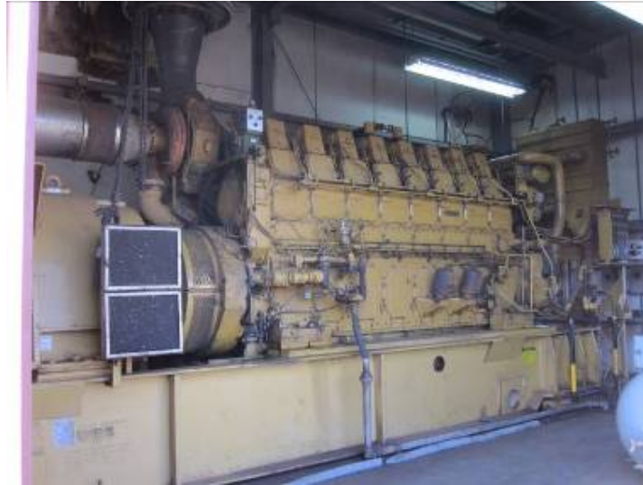
Figure 1-5. 2.2 MW diesel generator on Lanai, Photo by J. Keller, NREL
