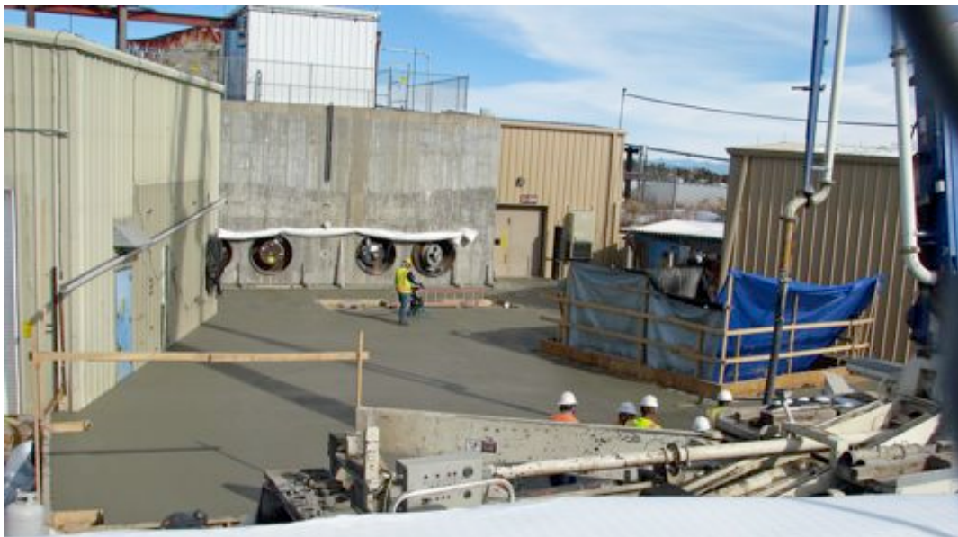
Figure 45: The WNR south yard after the concrete slab was poured on December 29 2012.
