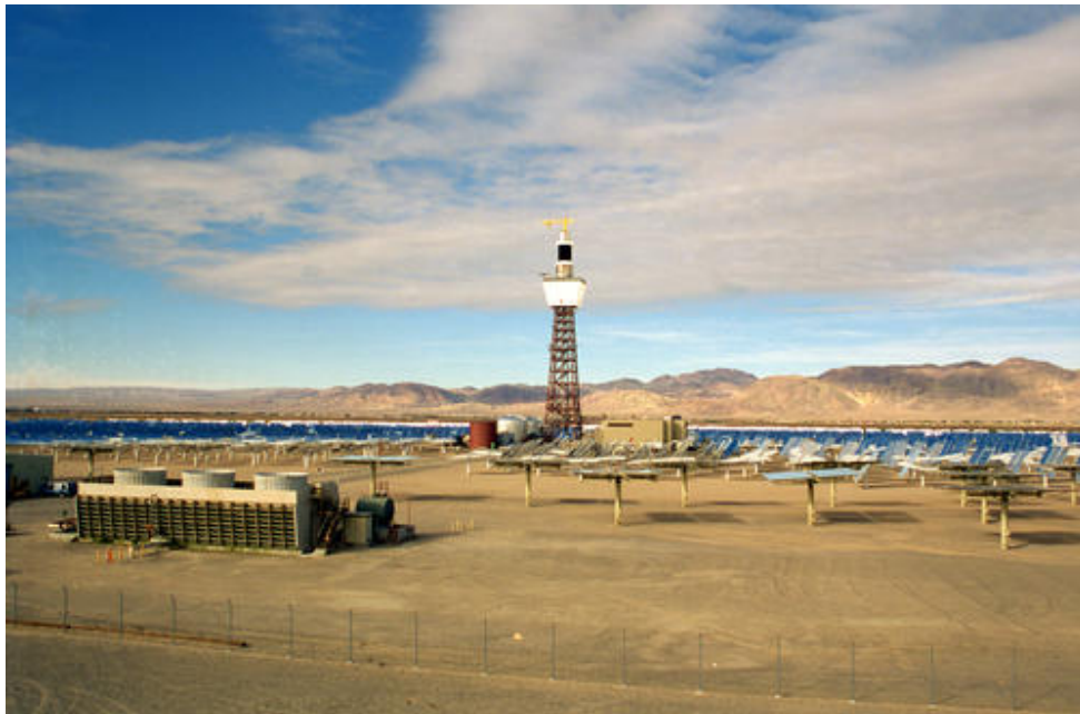
Figure 2-7. Aerial view of Daggett, California, DOE solar demonstration power tower. Photo by Joe Flores, NREL 02163
