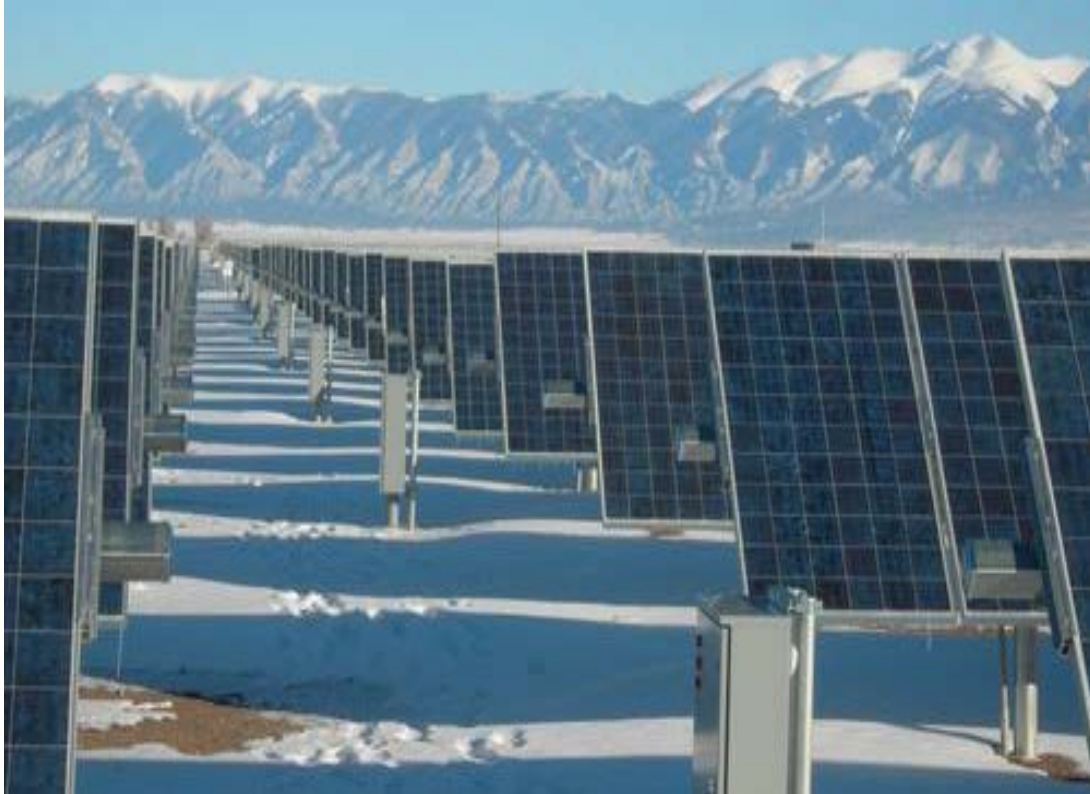
Figure 2-13. 8 MW, single-axis tilt-PV system in Alamosa, Colorado. Photo by Tom Stoffel, NREL 15558
