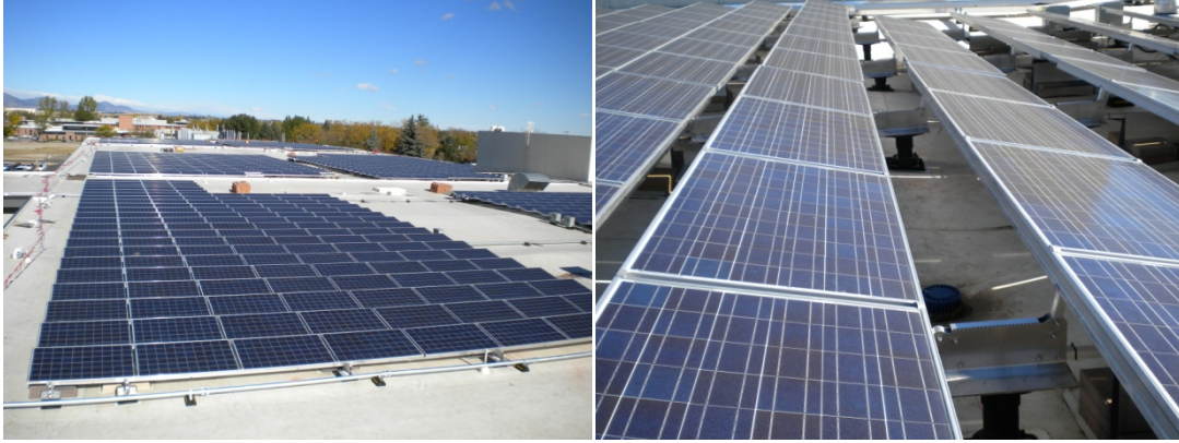
Figure 5-6. Typical ballasted PV system at GSA Denver Federal Center (Phoenix Area Office building roof PV would be similar). Photos by Otto VanGeet, NREL
