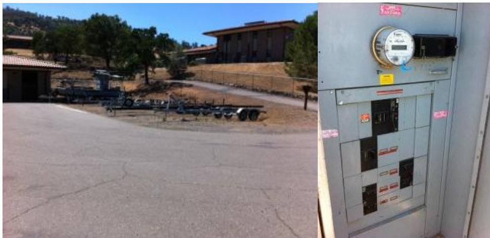
Figure 6-17. PV Carport Area 2: looking northeast (left), and main meter and electrical panel that serves south buildings at Lake Barryessa and possible PV tie in location (right). Photos by Otto VanGeet, NREL
