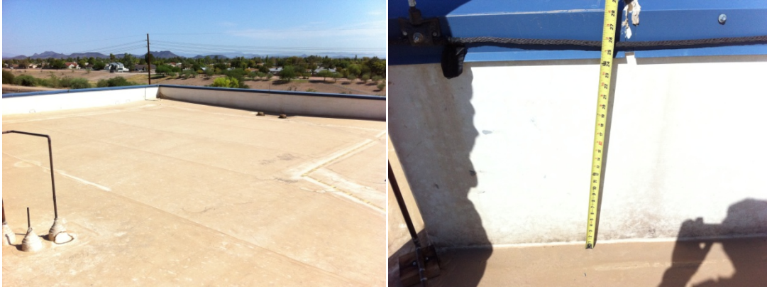
Figure 5-8. East wing roof looking east is also suitable for PV (left) and typical parapet is approximately 28” high (right). Photos by Otto VanGeet, NREL
