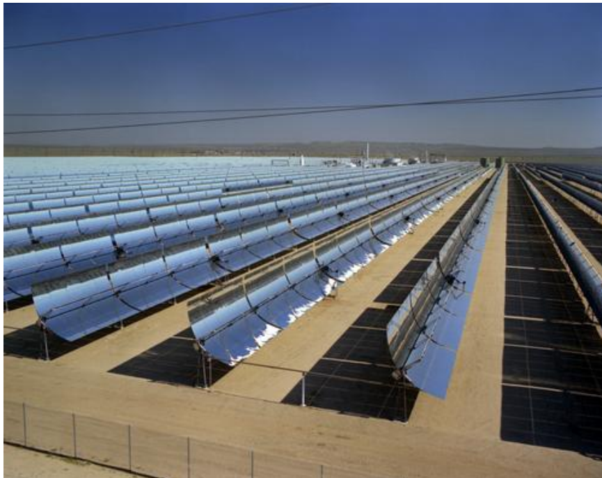
Figure 2-4. Aerial view of CSP trough plants at Kramer Junction, California (in operation for 30 years). Photo by Warren Gretz, NREL 01225
