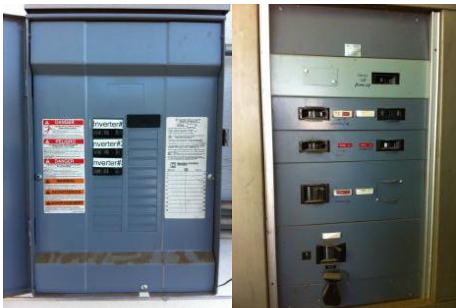
Figure 6-6. Existing PV system electrical breaker subpanel (left) and right building main 240 V, 600 A electrical panel with spaces for future solar breakers. Photos by Otto VanGeet, NREL
