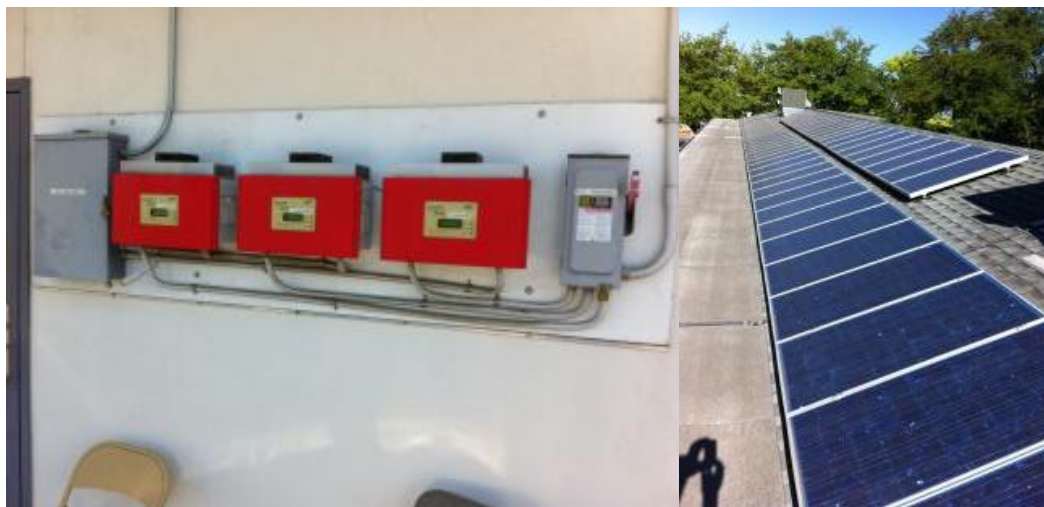
Figure 6-4. Existing inverters and PV system at Willows Office. Photos by Otto VanGeet, NREL
