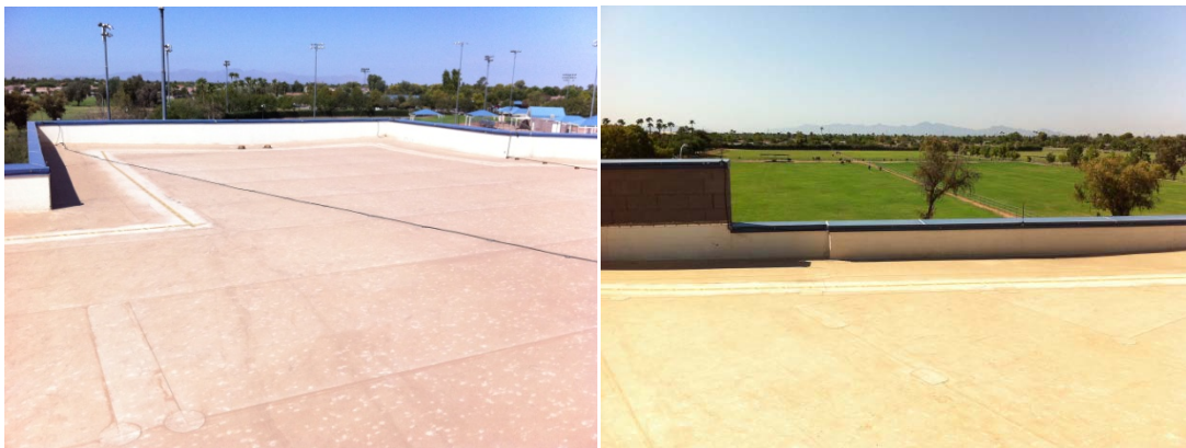
Figure 5-7. South wing looking west where PV is proposed (left) and looking south (right). Photos by Otto VanGeet, NREL
