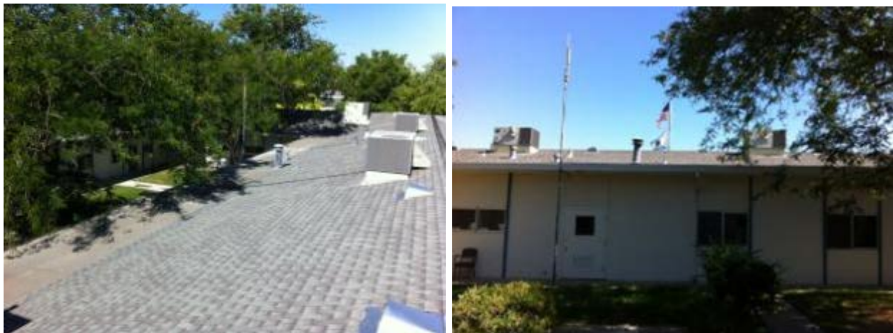
Figure 6-8. South-facing courtyard roof of Willow building looking west (Area 2) (left) and south-facing courtyard roof looking north from courtyard (right). Photos by Otto VanGeet, NREL
