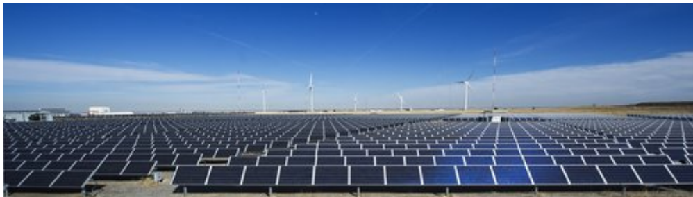
Figure 2-14. Photovoltaic field at the National Wind Technology Center. Photo by Dennis Schroeder, NREL 19794
