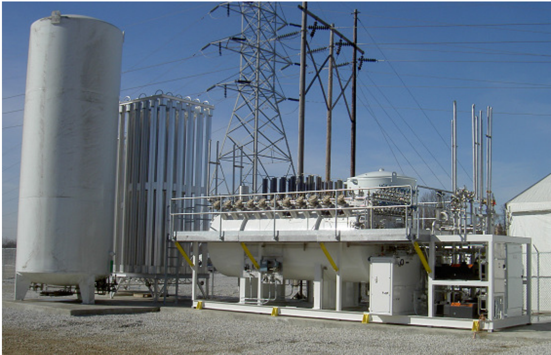
Figure 4. Open cycle cooling system utilized at the HTS Triax™ cable in Columbus, OH.
