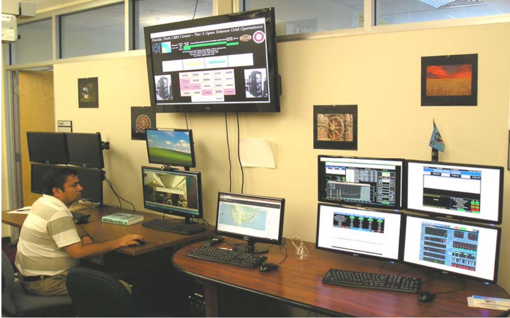
Fig. 4: Florida Tech Center for Tier-3 Open Science Grid Operations installed in 2011.
