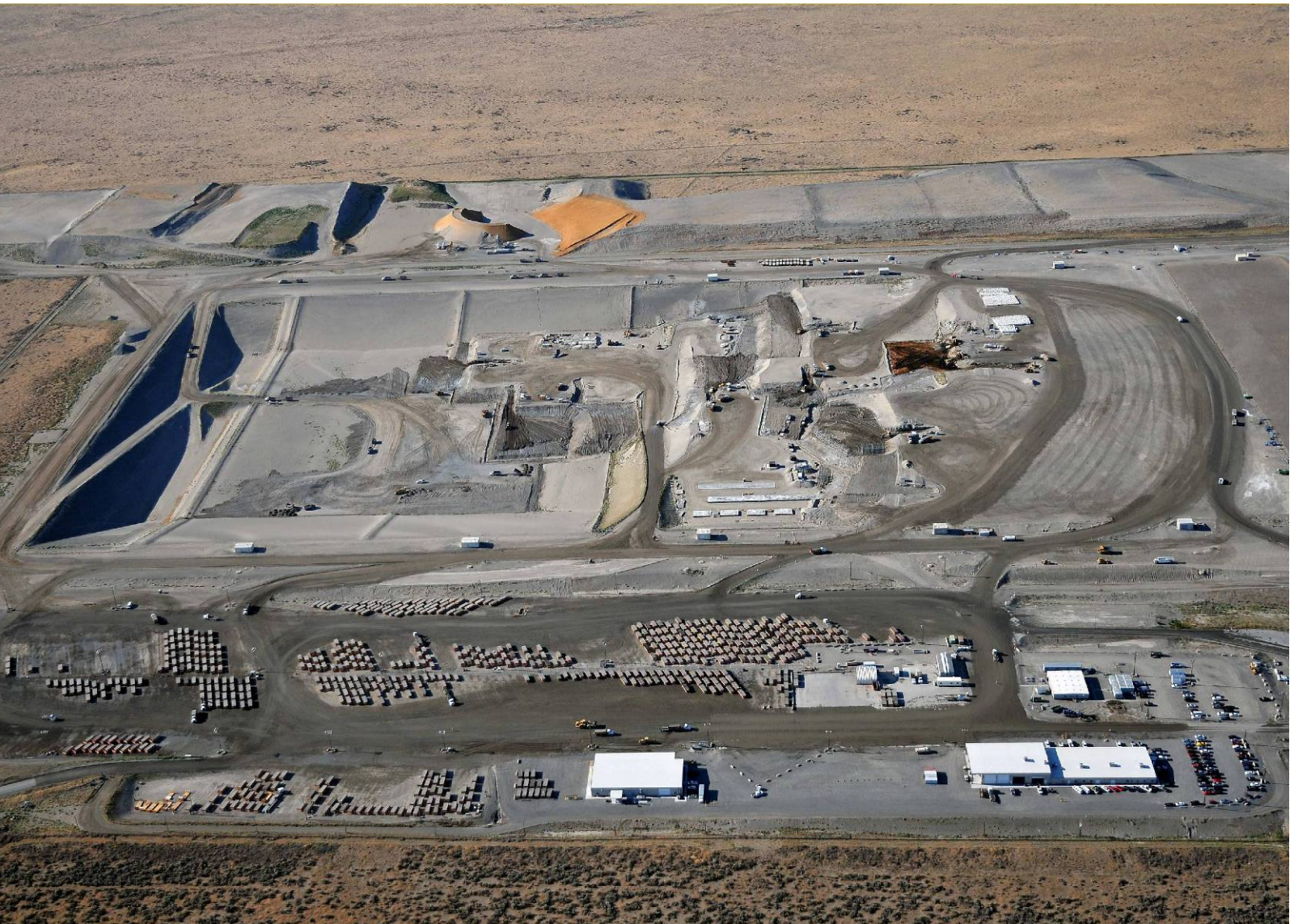
Figure 1. Aerial View of ERDF.
