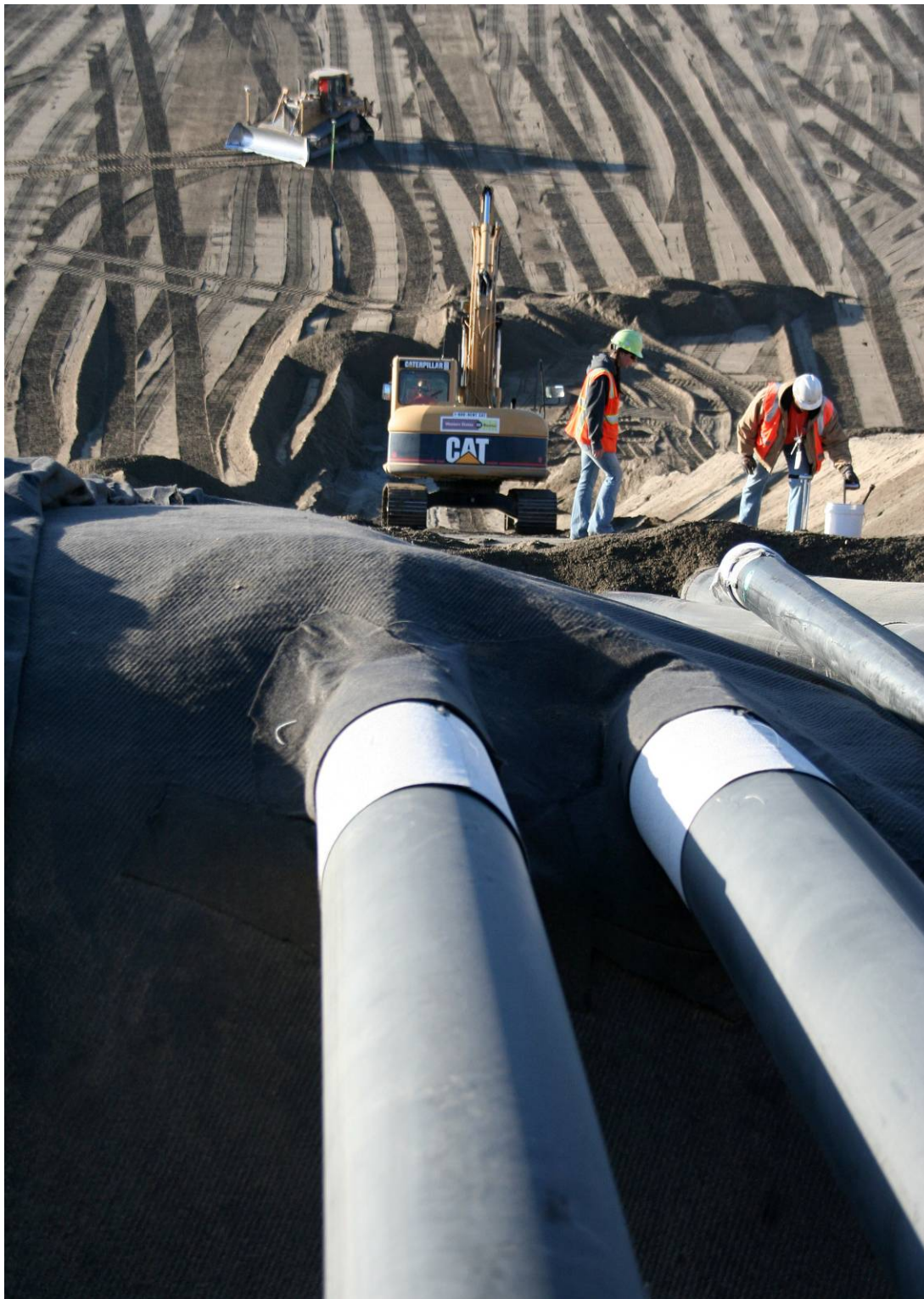
Figure 6. WCH Installs Leachate Transmission Pipes from the Super Cell 9 Sump to its Associated Crest Pad Building.
