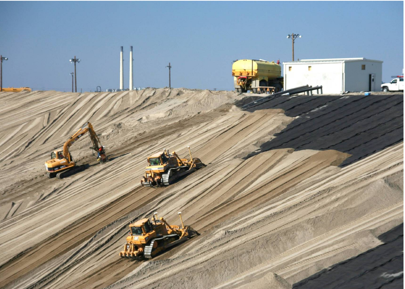
Figure 7. Each Super Cell Requires Only One Crest Pad Building.
