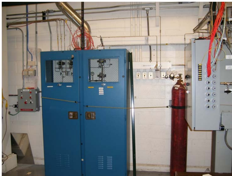
Figure 10. Gas Cabinet for Toxic Gas Cylinders Storage and PLC Box.
