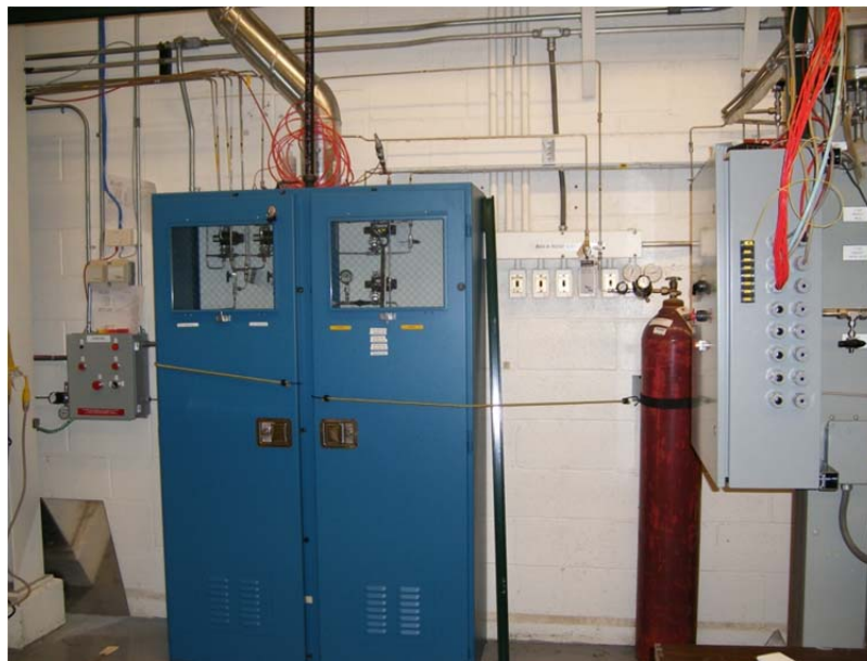
Figure 3.10 Gas Cabinet for Toxic Gas Cylinders Storage and PLC Box
