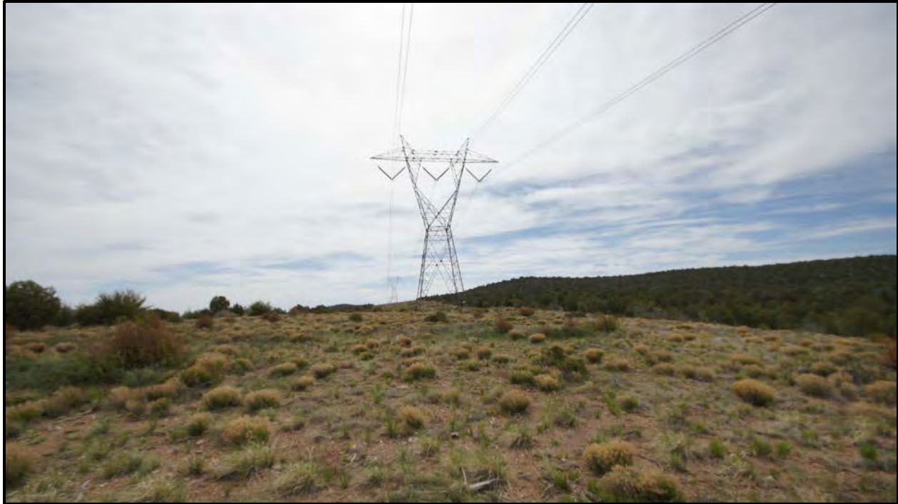
Figure 8. Four Corners-Moenkopi-Eldorado 500-kV line crossing the southern tip of the Clay Springs Wind Energy project area.
