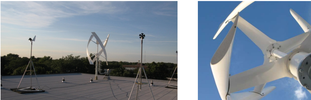
Figure 3. Wind turbine and anemometers with vanes on roof of SUL building.
