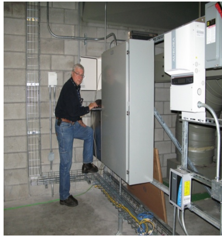
Figure 4: Electrical panel below wind turbine.
