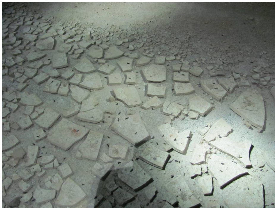
Figure 4. Bat Guano on Clearwell Floor.
