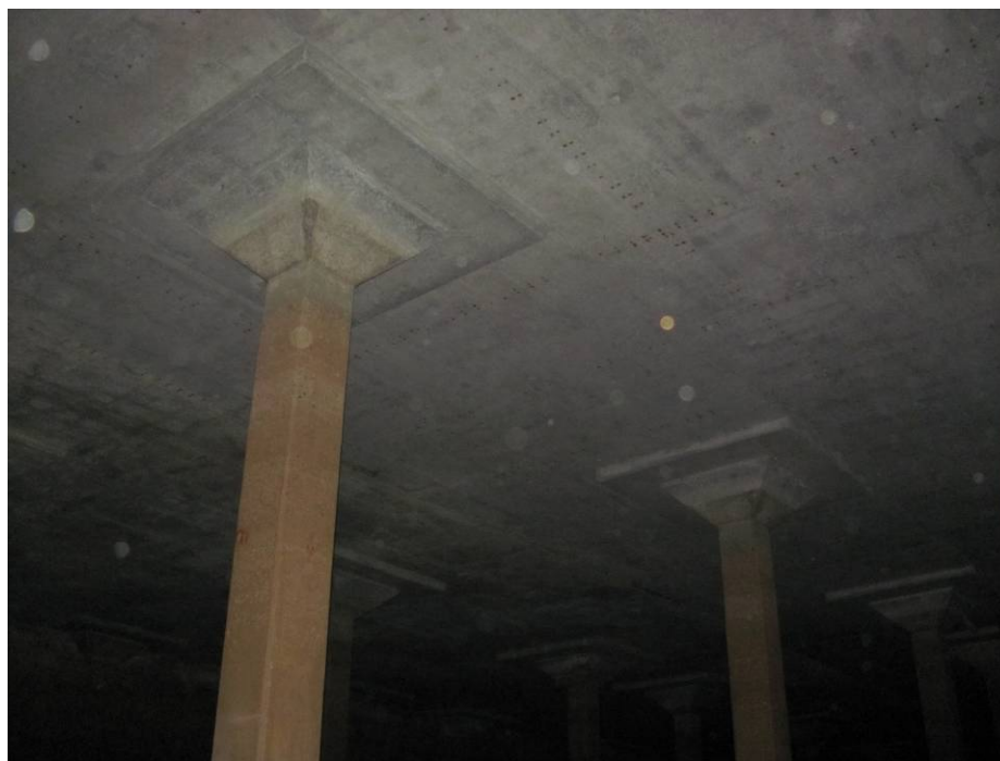
Figure 5. Typical Clearwell Roof Support Columns (no urine staining observed to indicate roosting).
