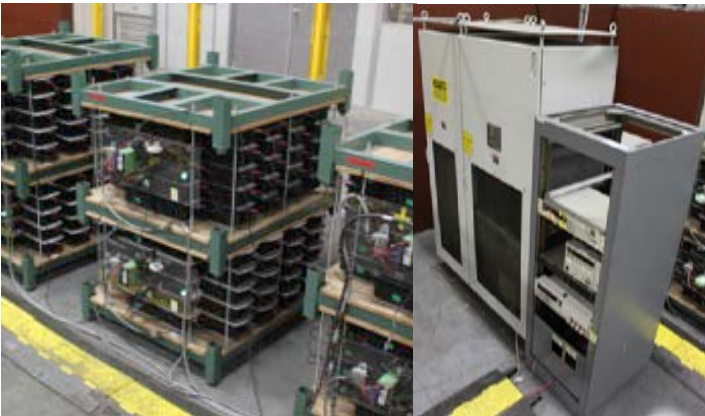
Figure 5 - DOE Test System at Aquion Headquarters
