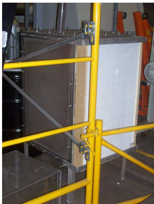
Figure 4: HEPA filtration system
