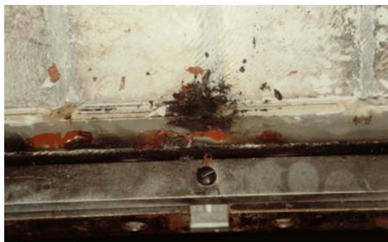
Figure 15. Burned Spot on the Heat Exchanger Created by Thermocouple Short.
