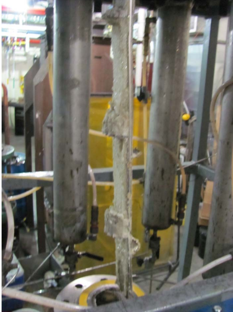
Figure 17. Internal baffles of gasifier quench pot No. 5 coated in tar.
