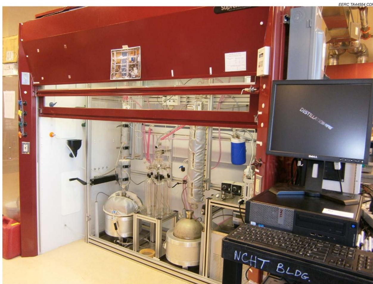
Figure 39. Distillation columns installed for DCL liquids separation.
