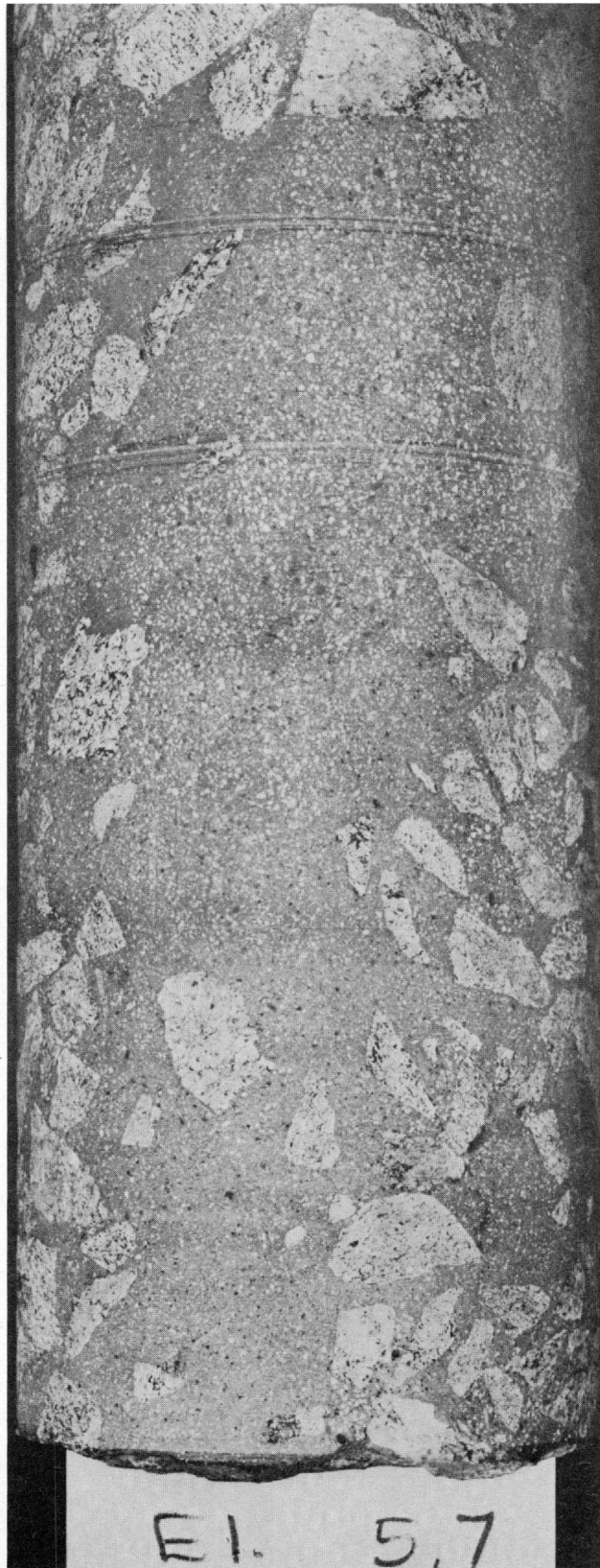
Close-up of section of core 2, near depth of 5.7 ft from top of pier, showing void in coarse aggregate
