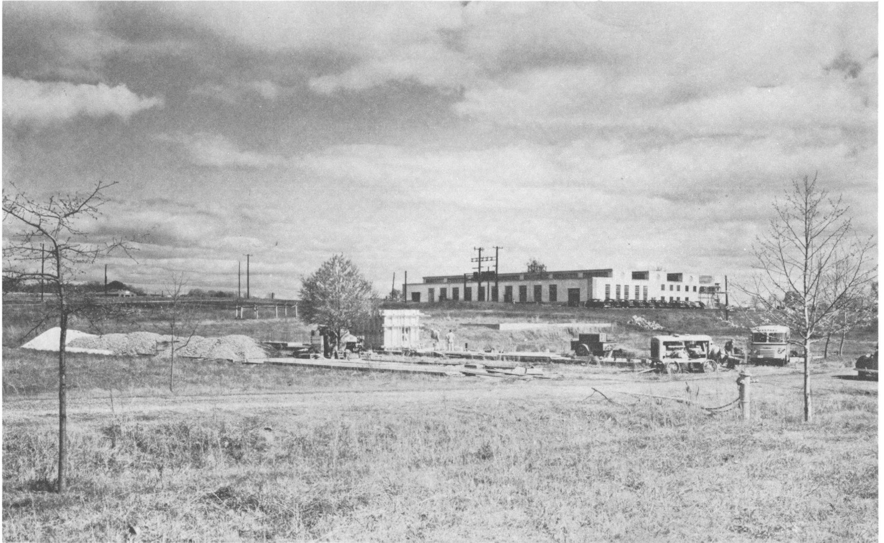
View of work area showing aggregate stockpiles, large block form under construction, and laboratory building in background
