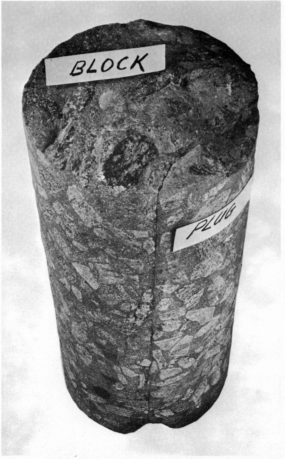
Section of core of Prepakt block to Prepakt plug at elevations 3.0 ft to 4.9 ft with 4.9-ft plane up, showing lack of bond between block and plug
