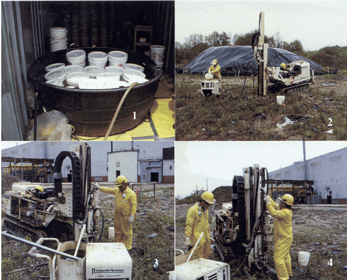
Figure 4. HRC injection – (1) Buckets are heated in a water bath; (2) HRC is transferred to the injection pump hopper; (3) The rod is driven to the required depth; (4) HRC is pumped through the rod as it is extracted.
