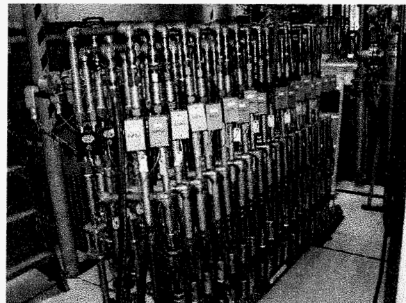
Fig. 6. Ion source cooling water supply and return manifolds and connecting hoses.
